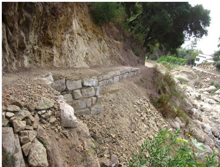
Photograph 6. Cut Sandstone Blocks on the Don Wall on the Cold Spring Trailhead
