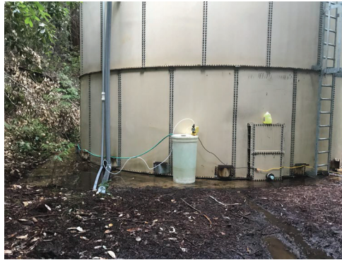
Figure 1. Temporary Disinfectant Injection Configuration at Well # 4
