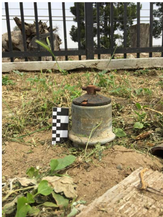
Photograph 2: Close-up of the Irrigation Valve.
