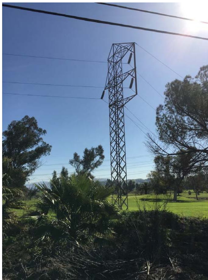
Overview of P-36-013627, within the El Prado Golf Course and south of Pine Avenue, facing south.
