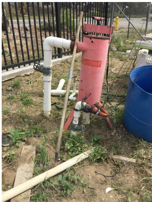
Photograph 3: Close-up of the Well Pump.
