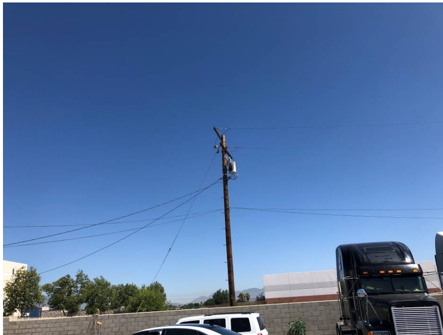
Pole-mounted transformers were observed along the north property of the Subject Property.
