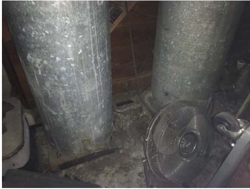
#37 WELL PRESSURE TANKS
