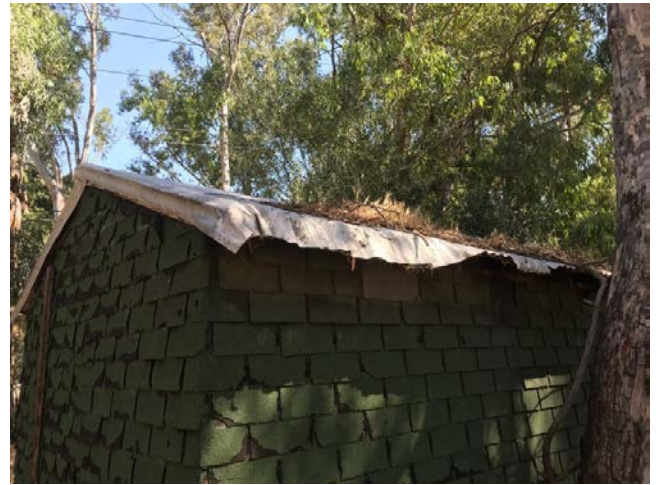
Suspect ACM roof and shingle siding office
