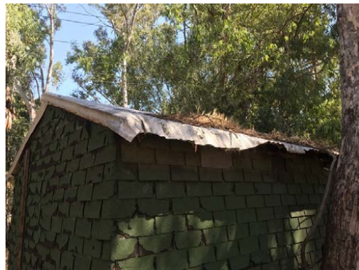
#48 SUSPECT ACM ROOF AND SHINGLE SIDING OFFICE
