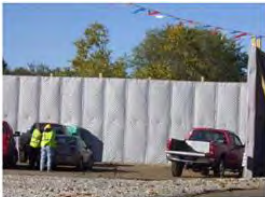
Figure 3 Substantial Temporary Construction Noise Barrier
