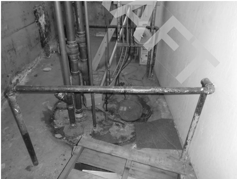
8. Sump pump in the basement
