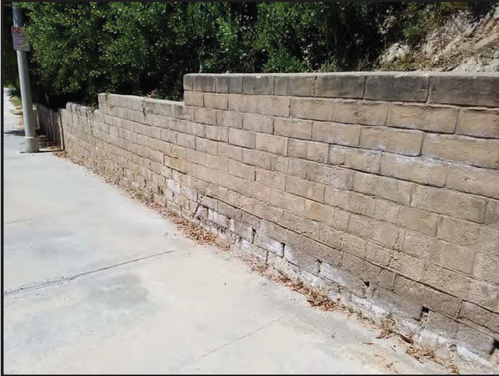
Photograph 2 – Northern Portion of Retaining Wall Condition (Note efflorescence and deterioration of CMU block)
