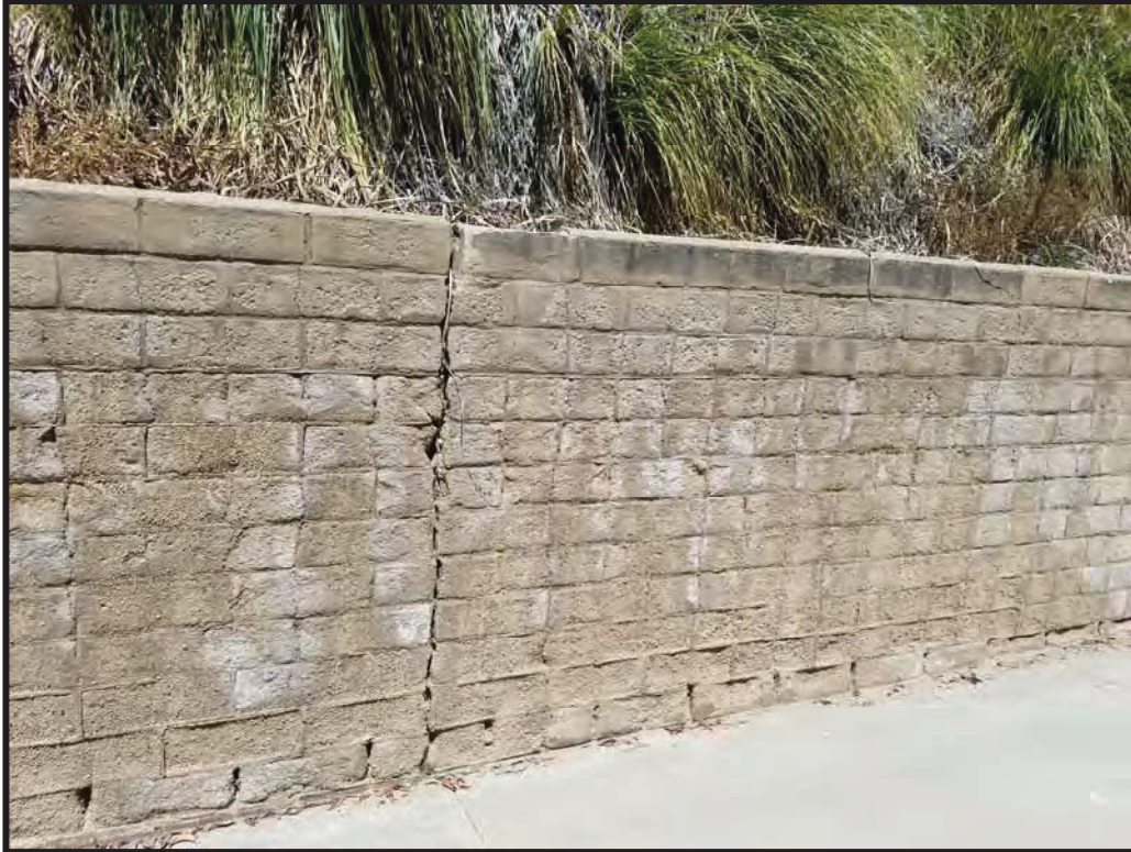
Photograph 4 – Retaining Wall Crack (Note efflorescence and deterioration of CMU block)
