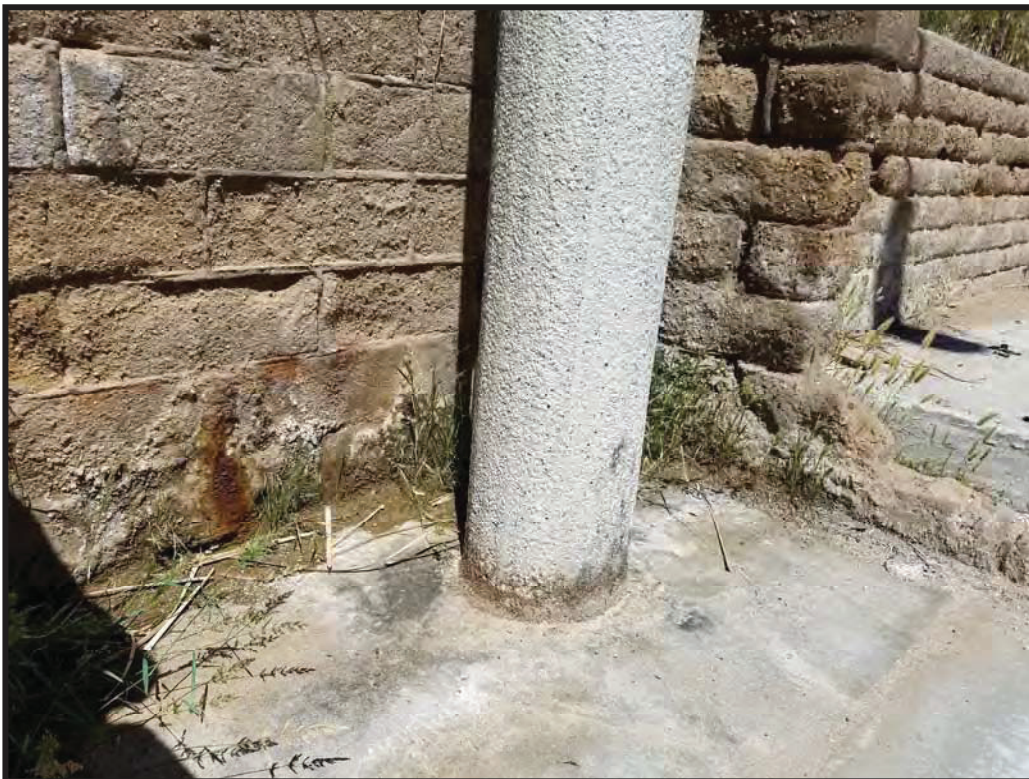
Photograph 5 – Retaining Wall Seepage near Park and Marina (Note corrosion, efflorescence and deterioration of CMU block)
