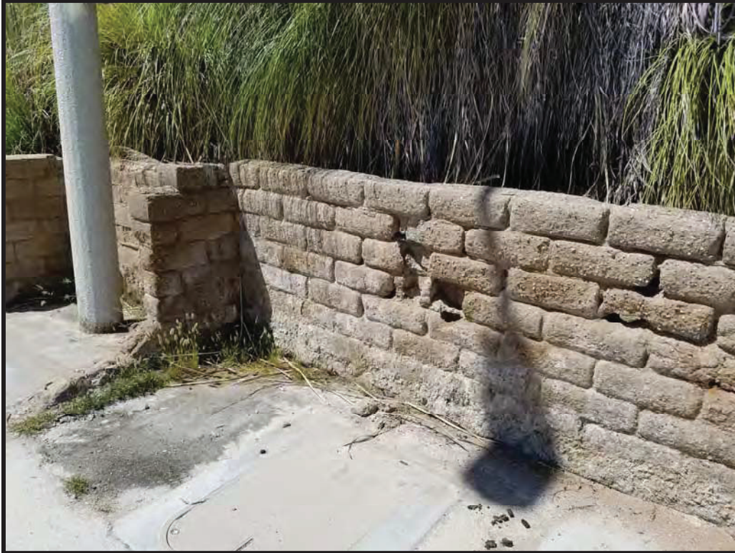
Photograph 6 – Retaining Wall Condition near Park and Marina (Note efflorescence and severe deterioration of CMU block)
