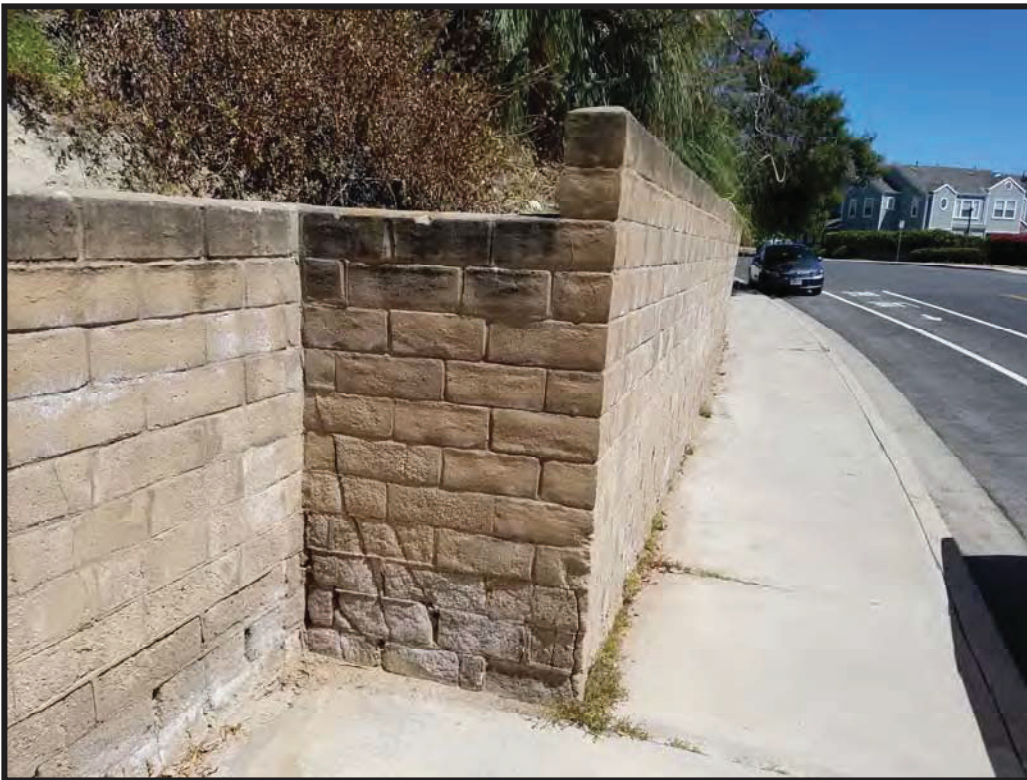
Photograph 3 – Retaining Wall Condition (Note efflorescence and deterioration of CMU block)
