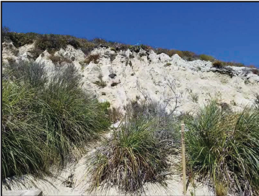
Photograph 7 – Looking East – Slope Face Erosion near Park and Marina
