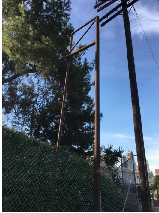
Photograph 3: Piping on-Site, looking southeast.
