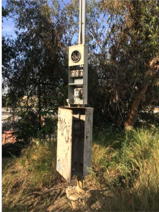
Photograph 5: Electrical Conduit on the central portion of the Site, looking southwest.
