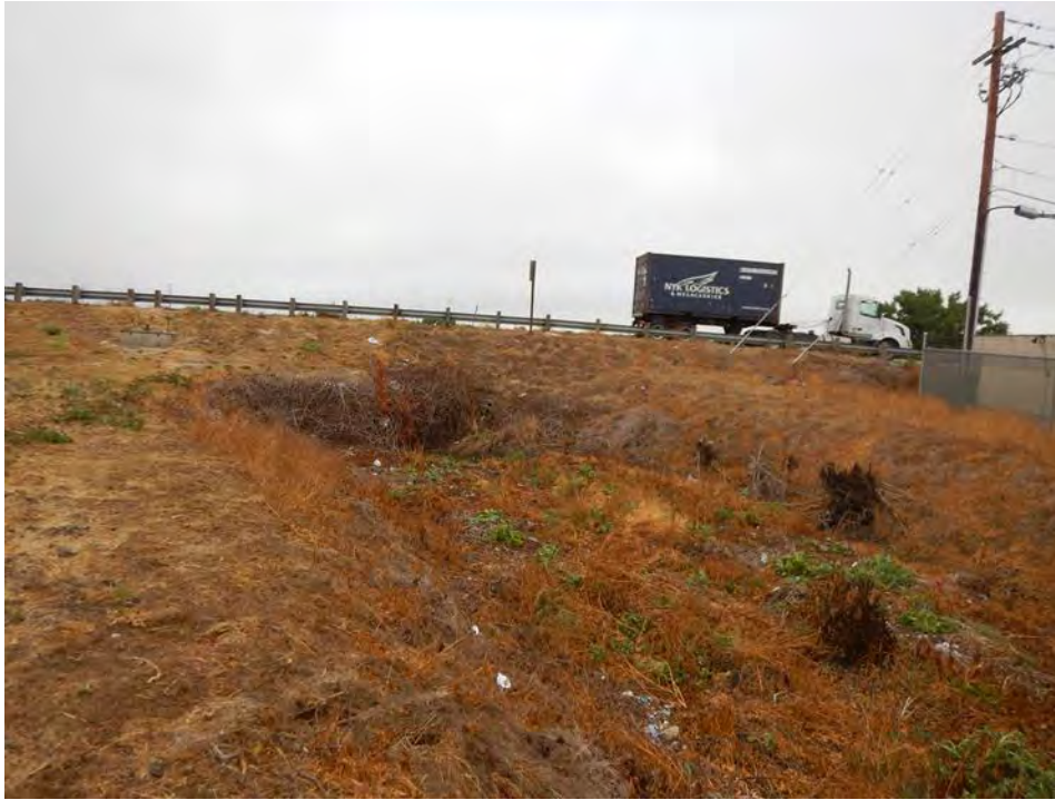
PP-1A Looking north at outflow point of culvert. Start of Lower Miller Slough
