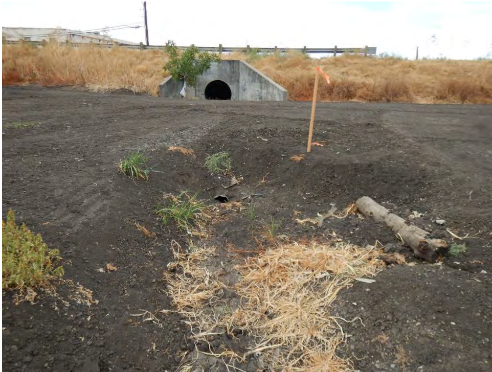
PP-8 Looking south at wetland swale 12 inch culvert and larger roadside ditch culvert in background.
