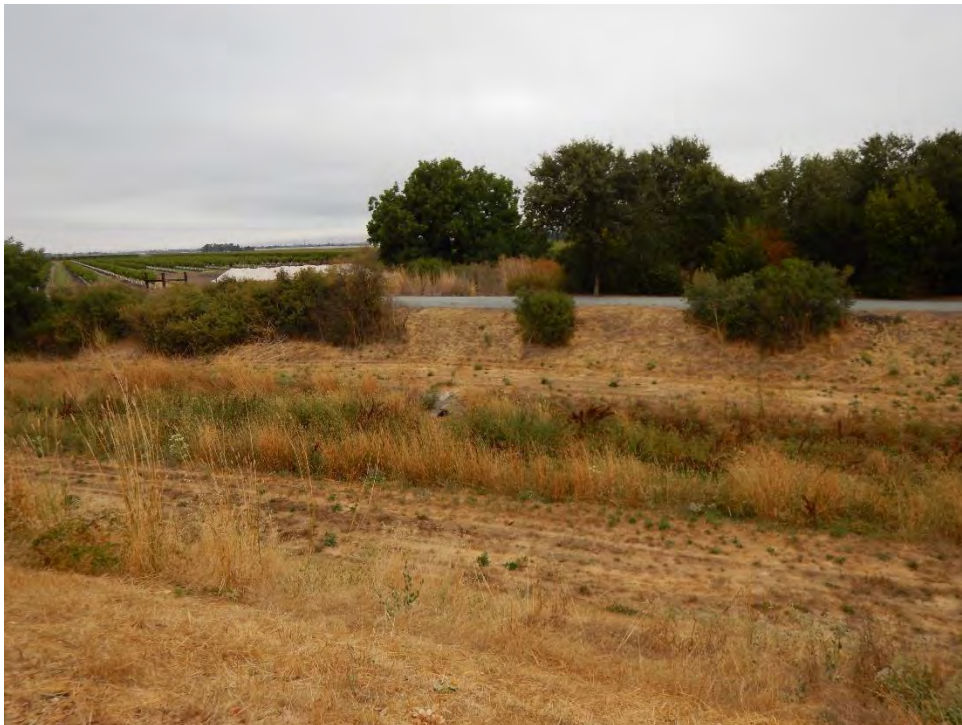
PP-4A looking north at Miller Slough/Llagas Creek and culvert on north side.
