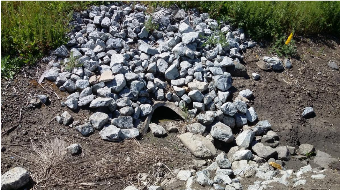
Photo #19: Southeast corner of the property facing east towards a stormwater inlet.
