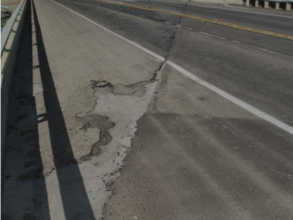
Asphalt concrete cracking at an abutment can be seen in this image.
