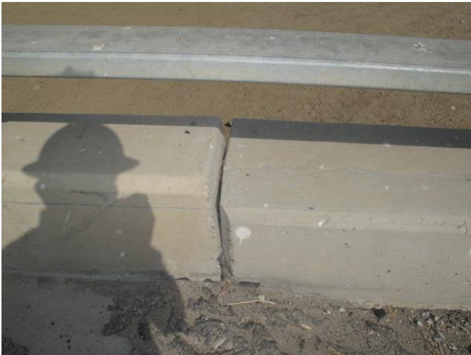
Displacement of the rail at an abutment can be seen in this image.
