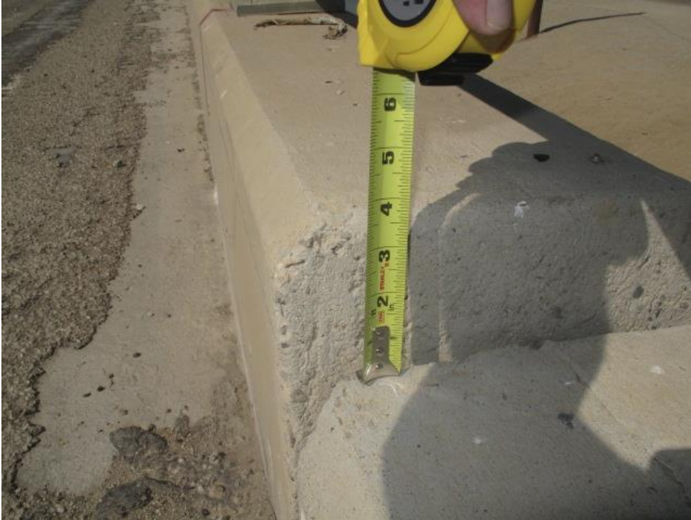
Vertical displacement of the rail at an abutment can be seen in this image.
