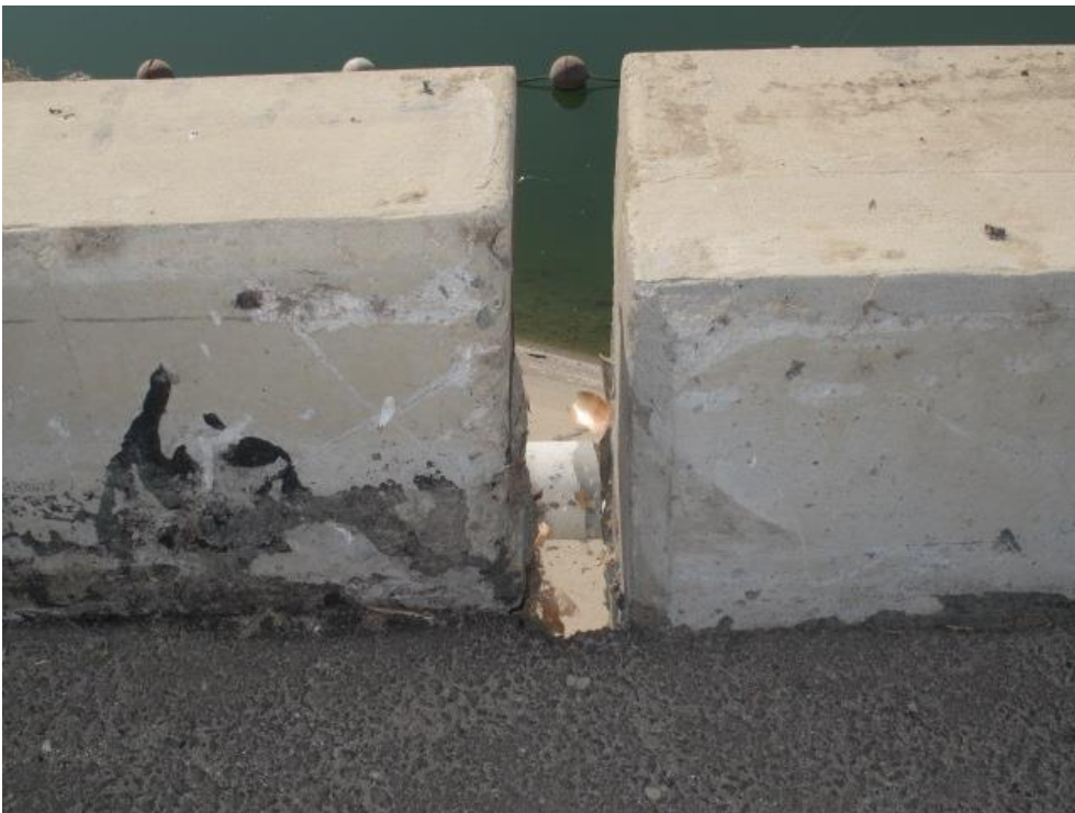
Horizontal displacement of the rail at an abutment can be seen in this image.
