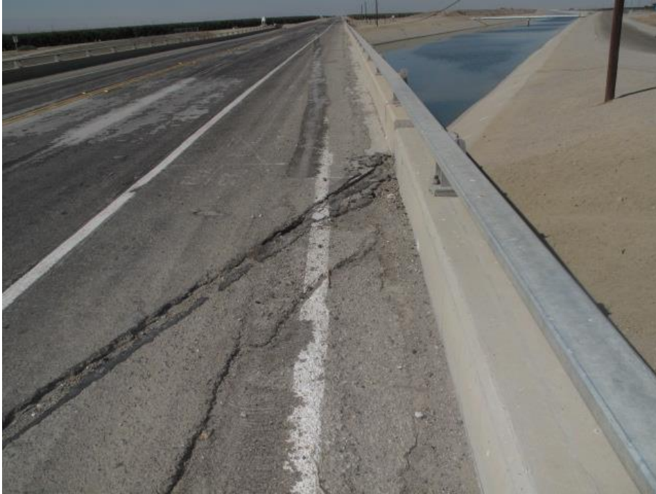
Asphalt concrete cracking at an abutment can be seen in this image.
