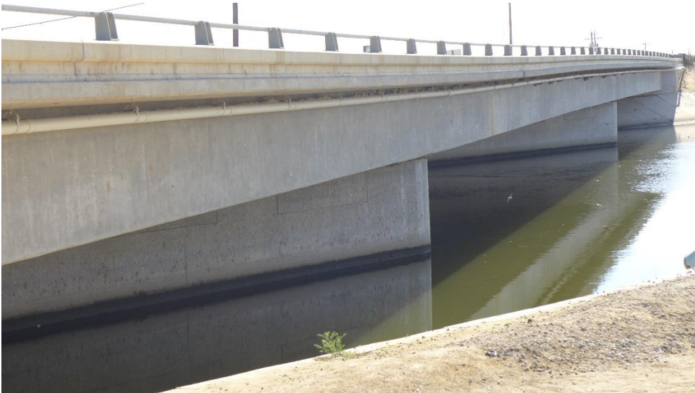
The bridge deck is sagging and is no longer visibly level in this image.
