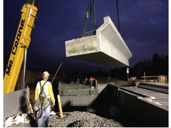
Overhead protection is required when moving heavy objects over Metro ROW or in areas designated for public use.
