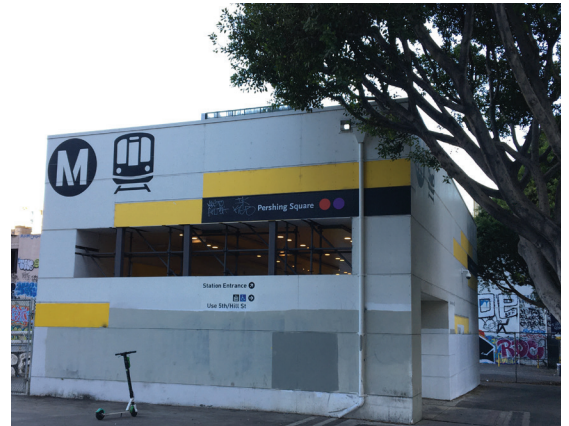
Constructed above is a wooden box over the entrance portal for overhead protection at the 4th/Hill Station.
