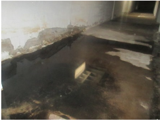
#81 MOISTURE CONDITION IN BASEMENT OF 499 BUILDING
