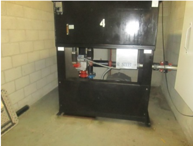
Hydraulic elevator equipment in parking garage
