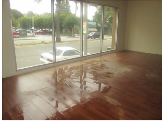
#80 MOISTURE CONDITION IN GROUND FLOOR OF 499 BUILDING
