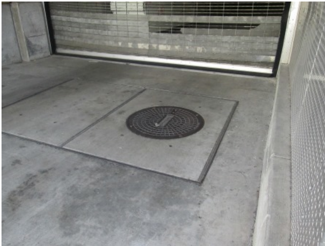
Vaulted transformer on northwest exterior of 441-483 Building
