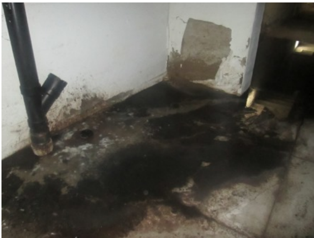
Moisture condition in basement of 499 Building
