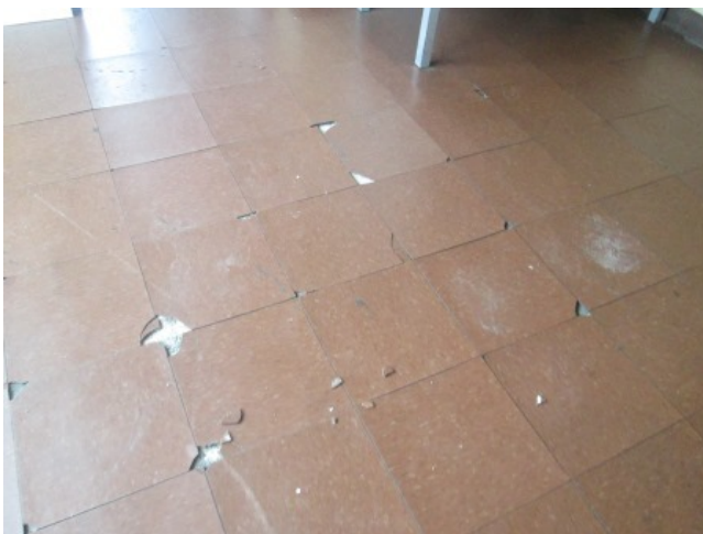
Damaged vinyl floor tile in second floor of 577 Building
