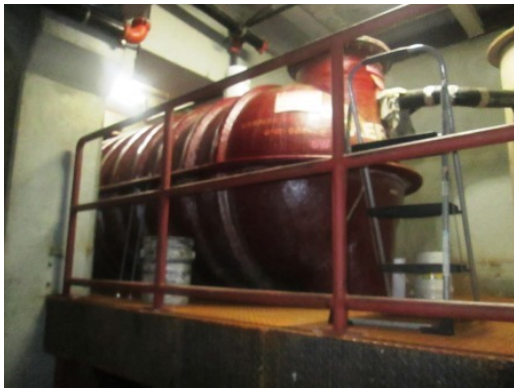
#63 GREASE TRAP IN PARKING GARAGE OF 441-483 BUILDING (WHOLE FOODS)
