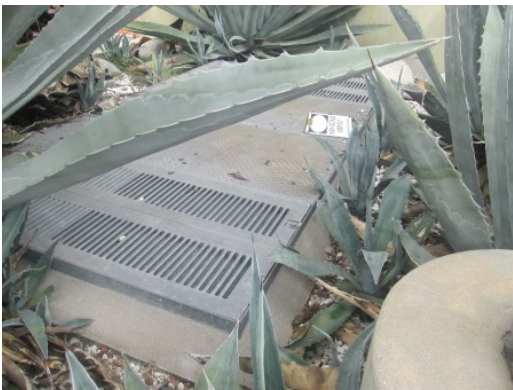
#54 VAULTED TRANSFORMER ON WESTERN EXTERIOR OF 577 BUILDING
