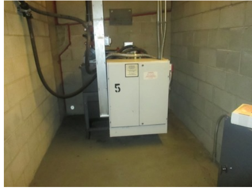
#56 HYDRAULIC ELEVATOR EQUIPMENT IN PARKING GARAGE
