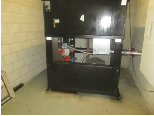
#55 HYDRAULIC ELEVATOR EQUIPMENT IN PARKING GARAGE
