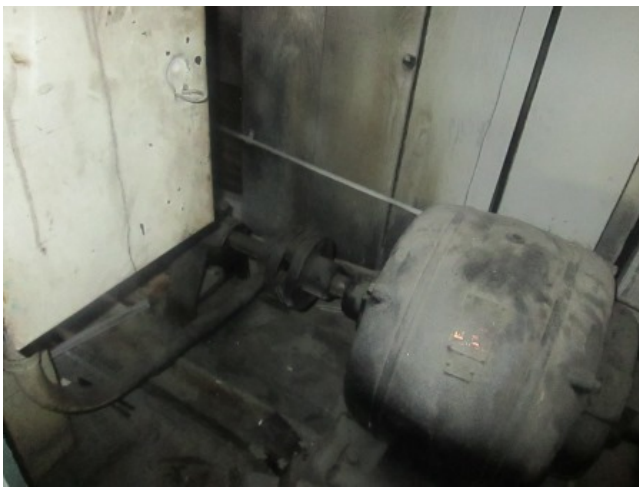
Hydraulic lift equipment in the basement of the 499 Building
