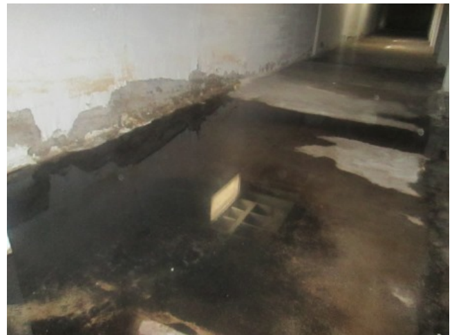
Moisture condition in basement of 499 Building
