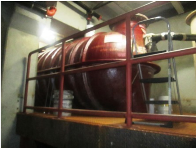
Grease trap in parking garage of 441-483 Building (Whole Foods)
