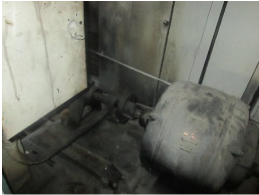
#57 HYDRAULIC LIFT EQUIPMENT IN THE BASEMENT OF THE 499 BUILDING
