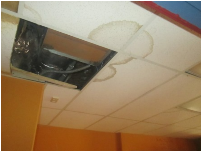
Evidence of moisture condition in second floor ceiling of 577 Building
