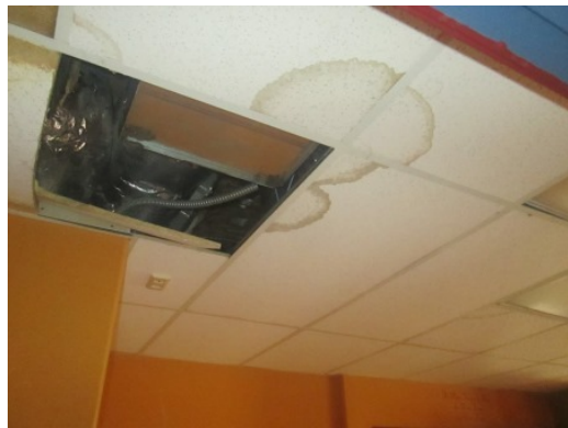
#84 EVIDENCE OF MOISTURE CONDITION IN SECOND FLOOR CEILING OF 577 BUILDING
