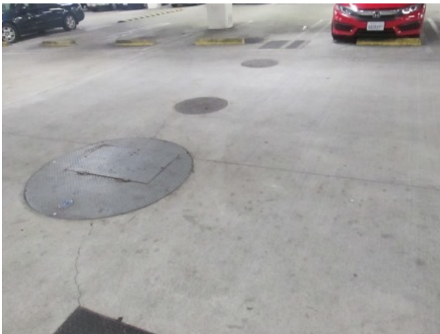
Sump and oil-water separator in parking garage of 441-483 Building
