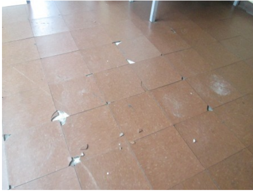
#79 DAMAGED VINYL FLOOR TILE IN SECOND FLOOR OF 577 BUILDING
