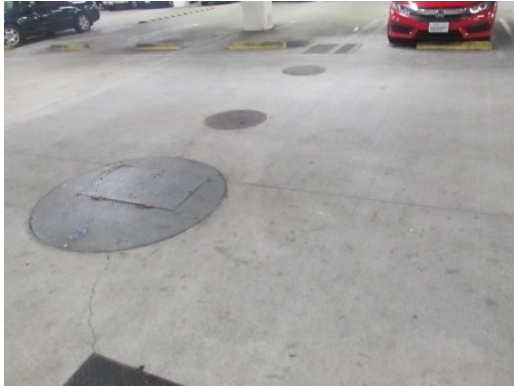
#67 SUMP AND OIL-WATER SEPARATOR IN PARKING GARAGE OF 441-483 BUILDING
