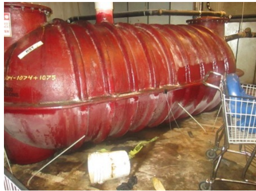
#64 GREASE TRAP IN PARKING GARAGE OF 441-483 BUILDING (WHOLE FOODS)
