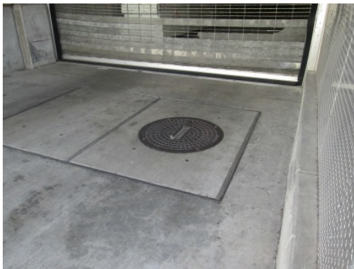
#53 VAULTED TRANSFORMER ON NORTHWEST EXTERIOR OF 441-483 BUILDING
