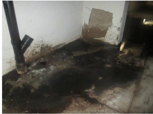
#82 MOISTURE CONDITION IN BASEMENT OF 499 BUILDING
