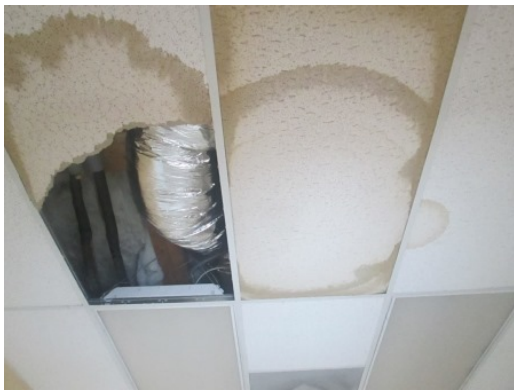
#83 EVIDENCE OF MOISTURE CONDITION IN SECOND FLOOR CEILING OF 577 BUILDING
