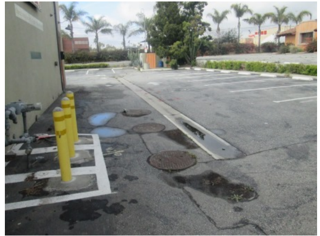
Below-grade grease trap on northern exterior of 577 Building
