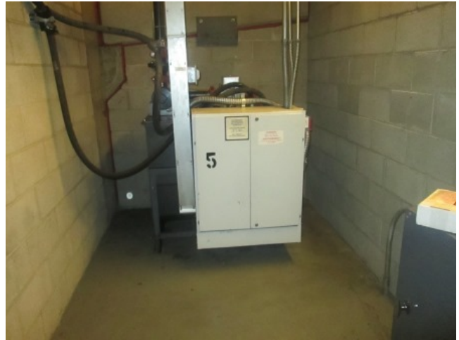
Hydraulic elevator equipment in parking garage
