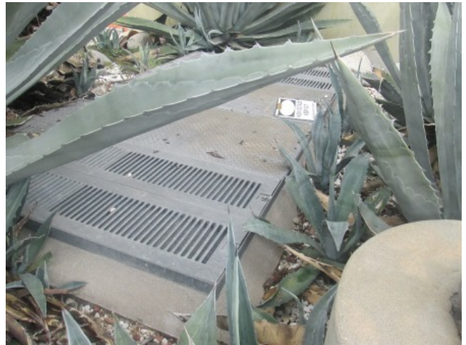
Vaulted transformer on western exterior of 577 Building
