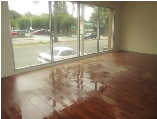
Moisture condition in ground floor of 499 Building
