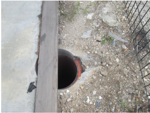
#69 OPEN PIPE ON NORTHWEST CORNER OF 441-483 BUILDING (WHOLE FOODS)
