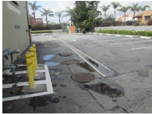
#62 BELOW-GRADE GREASE TRAP ON NORTHERN EXTERIOR OF 577 BUILDING
