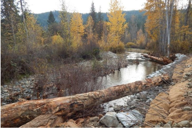
Figure 6-2: Engineered large wood installed in the lower reaches of East Weaver Creek in November 2014.
