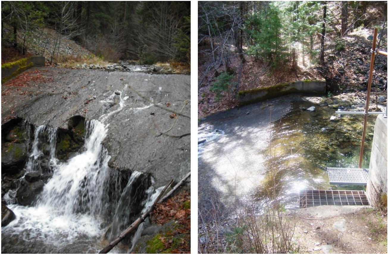
Figure 2-3. Dam showing concrete cap (left) and stilling basin to the EWF (right).
