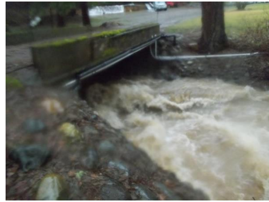
Figure 10-5: Butterfield Private Road Bridge in December 2015 (Above Left) and in January 2016 during an estimated Q2-Q4 storm flow.
