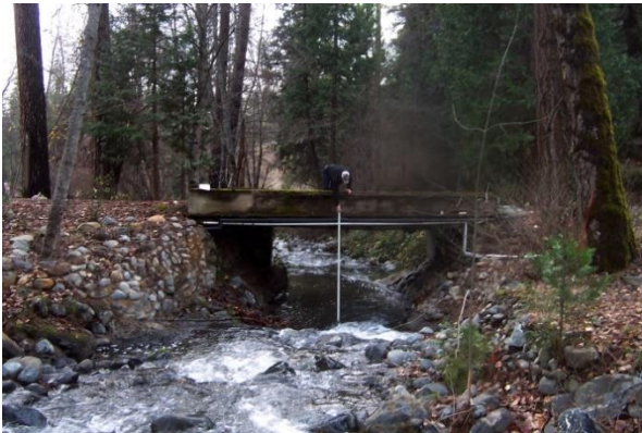
Figure 10-4: Butterfield Private Road Bridge shown in December 2015 is the most undersized crossing.
