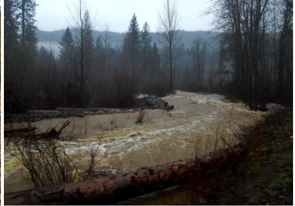
Figure 6-3: Engineered large wood installed in the lower reaches of East Weaver Creek in November 2014 during an approximately Q_7 flow in January 2016.
