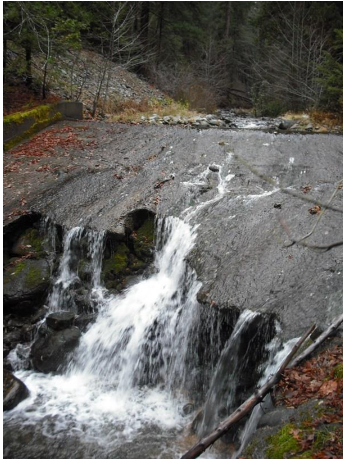
i: East Weaver Dam- integrity of the structure has been compromised by undercutting.
