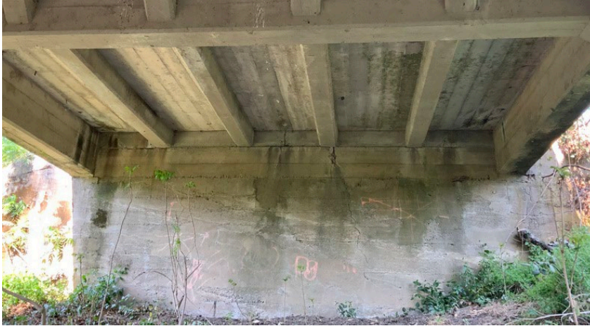
Photo 6: Looking eastbound at Abutment 2 displaying soffit cracks and vertical cracks (taken April 2021).
