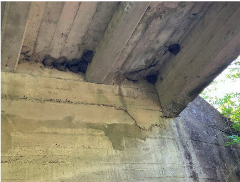
Photo 5: Looking westbound at Abutment 1 displaying spalls next to Girder 1 (taken April 2021).
