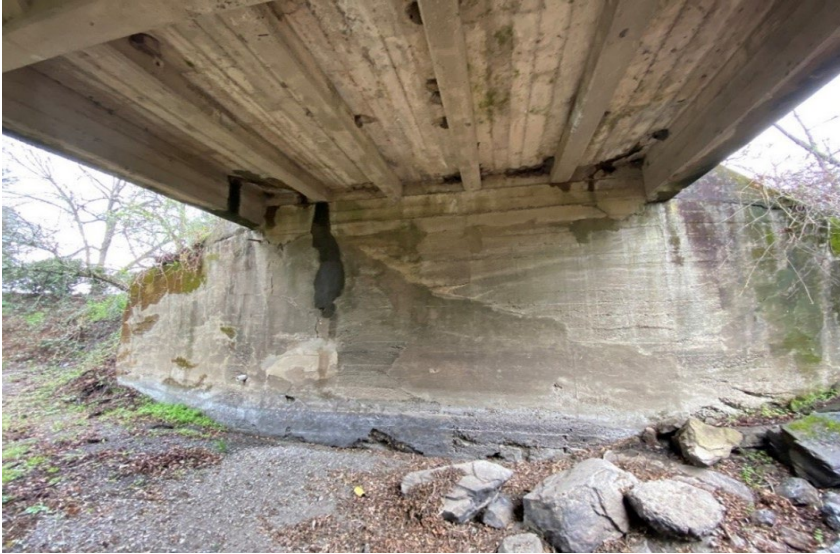
Photo 2: Looking westbound at Abutment 1 displaying patched and repaired concrete areas (taken in 2015).
