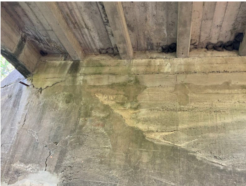
Photo 3: Looking westbound at Abutment 1 displaying the spall at the bottom face of Girder 2 (taken April 2021).
