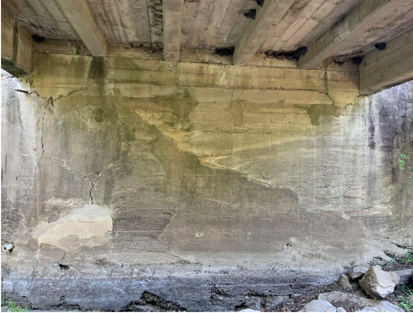
Photo 4: Looking westbound at Abutment 1 displaying multiple spalls in the face; Girder 2 (left), Girder 1 (right) (taken April 2021).
