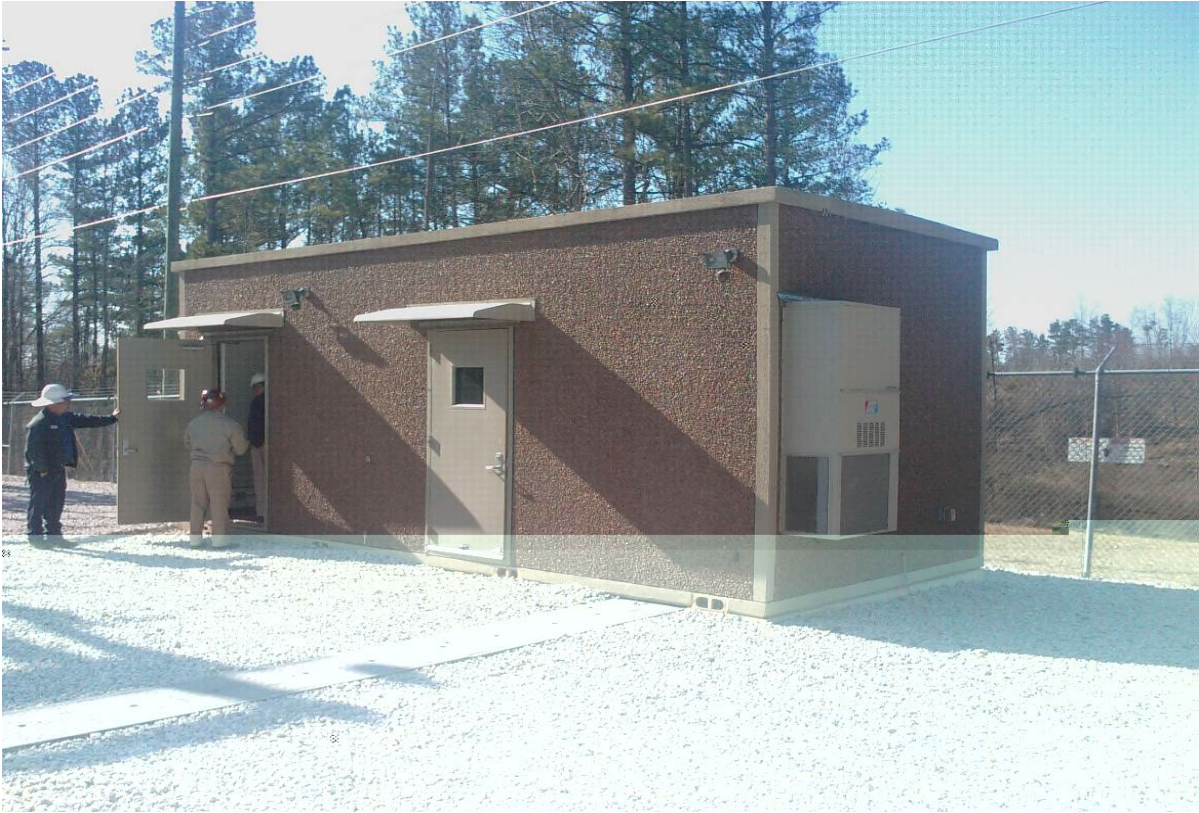
Figure 2-6. Typical Control Room
