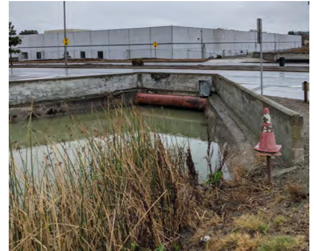
Stormwater management system in Moffett Park after King Tide event
