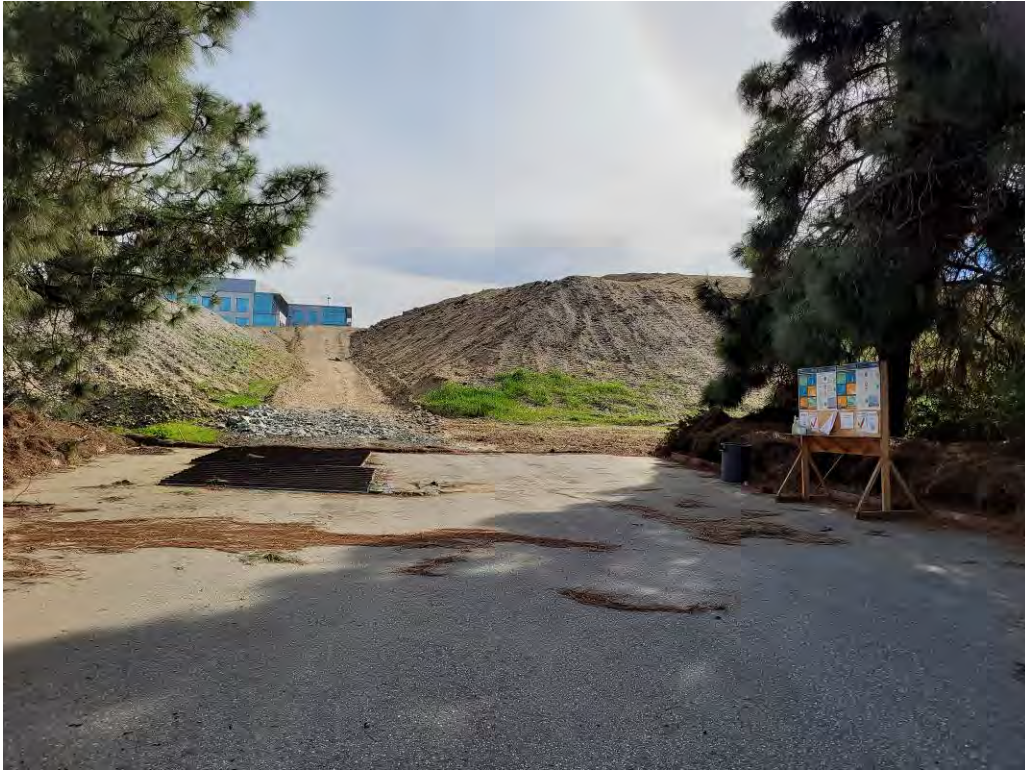
Photograph 9: East side of Geneva Drive between East Caribbean Drive and Caspian Drive, large stockpile.
