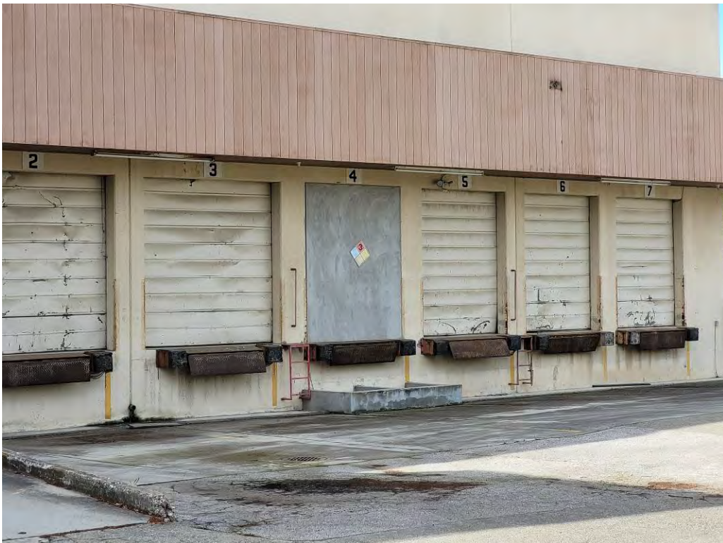
Photograph 4: 1319 Moffett Park Drive, hazardous materials sign and rolling doors.
