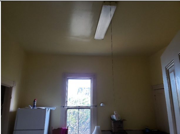
Photograph No. 15. View of fluorescent light in kitchen.
