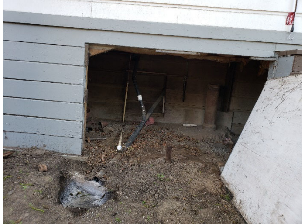
Photograph No. 14. View of leaking drainline at western portion of home.
