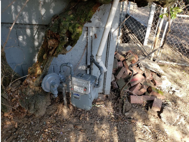
Photograph No. 25. View of gas meter.
