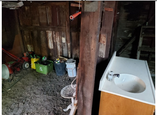
Photograph No. 18. View of House 3 kitchen with ACM sheet flooring and mastic.
