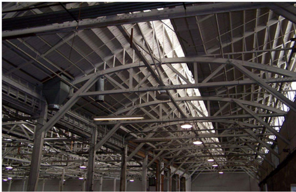
Figure 4-7. FMC Plant 1 Building A, Interior Bowstring Truss and Sawtooth Roof (Looking West/Southwest)
