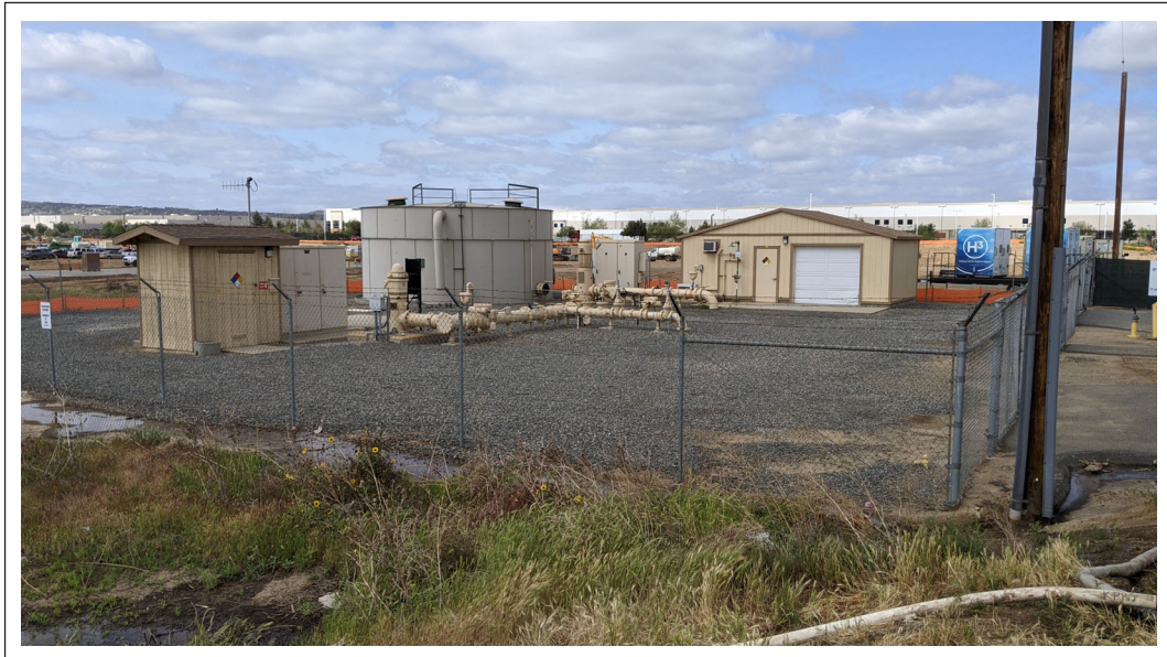
Photo of Well 56 facing southwest. Unrelated construction activities are occurring on adjacent parcel and puddled water in photograph are from actively leaking hoses used to fill construction water trucks.
