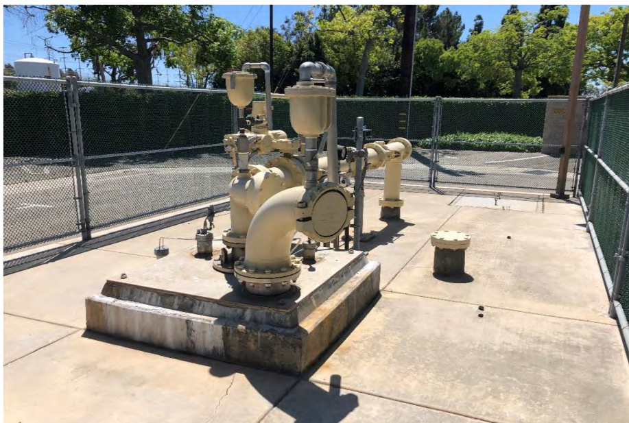
Photo 1: Example Injection Well Site
