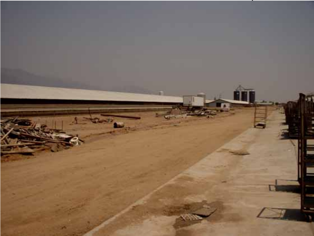
View of trash and metal debris to the west of silos.
