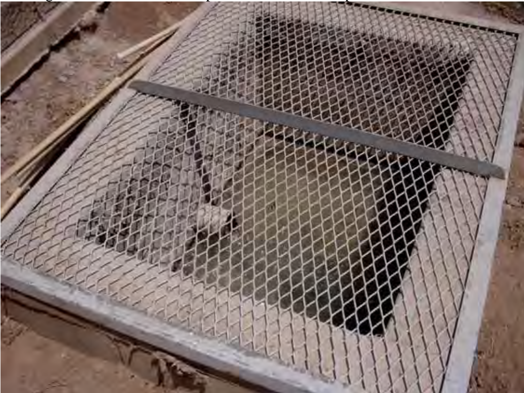
Small wastewater sump that is part of the wastewater collection system.
