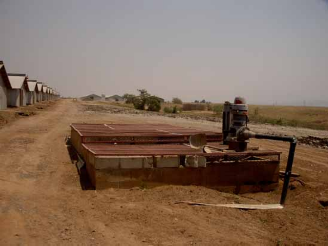
Looking east towards southeast corner of site with wastewater collection sump in foreground.
