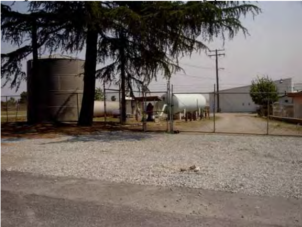
Looking south at production well near Cherry Valley Boulevard.
