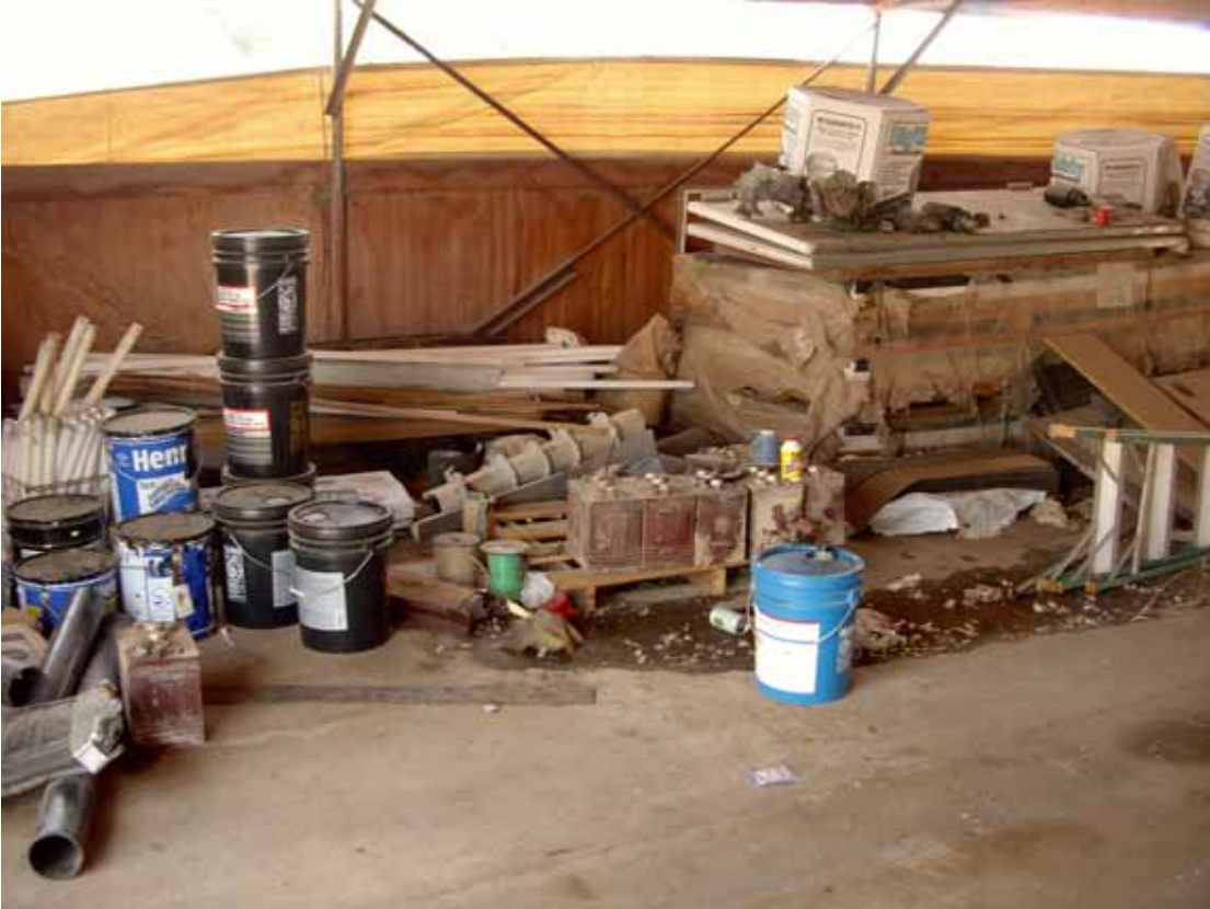
View inside diesel backup power room with spent batteries in center of picture.
