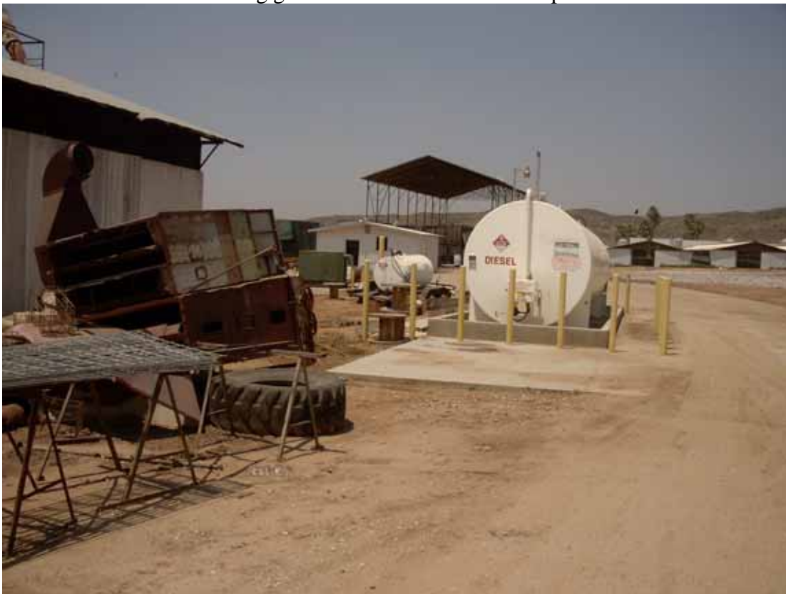
View to north of above ground storage tank for diesel.
