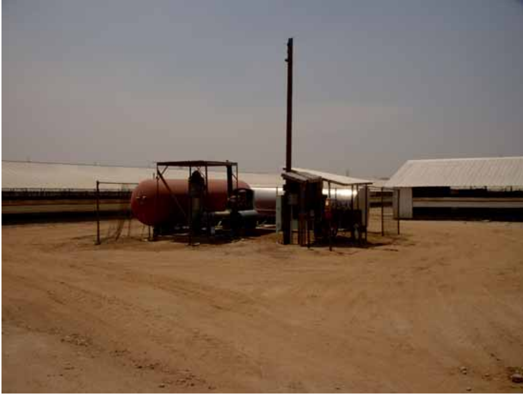
View to west showing groundwater production well and associated tanks at southeast portion of site.
