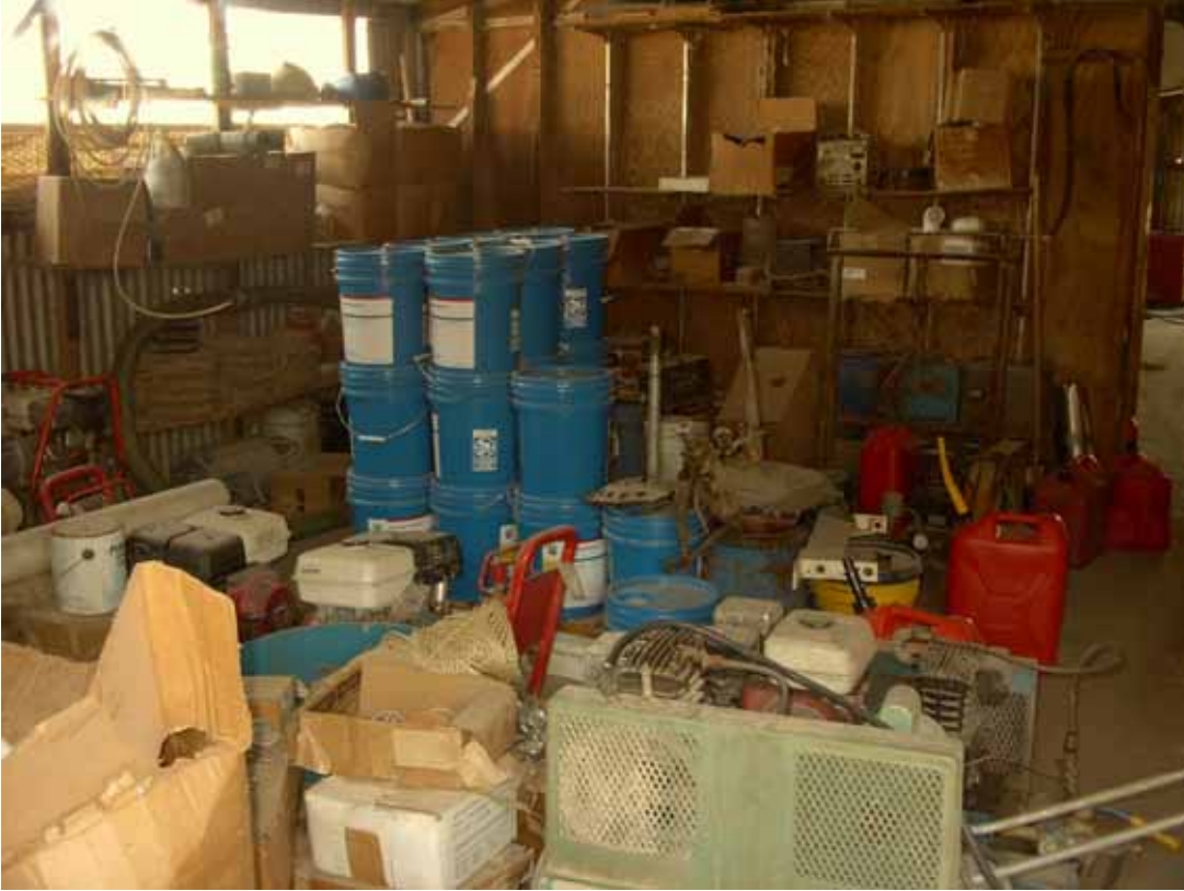
Additional view of contents inside mechanical building.
