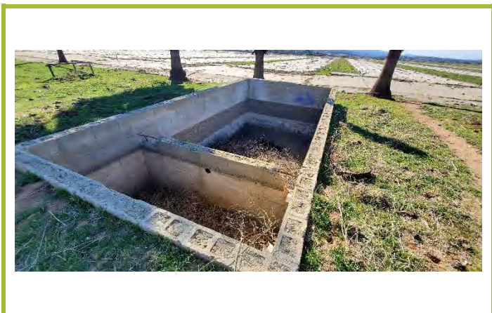
Photograph #17: View of sub-grade vaults on the central portion of the site.
