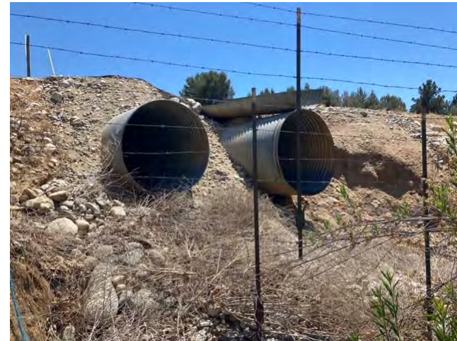
Photo 22. View of culvert outlets located along the southern extent of the review area under Brookside Avenue, facing south. Flows from the culvert outlets continue into NWW-3 (33.961603, -117.018517). June 3, 2021.
