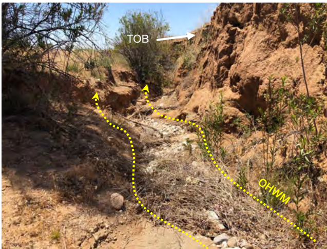
Photo 23. Downstream view of NWW-3, facing northwest, located just north of the two culvert outlets under Brookside Avenue before NWW-3 converges with NWW-3A (33.961636, -117.018604). June 3, 2021.
