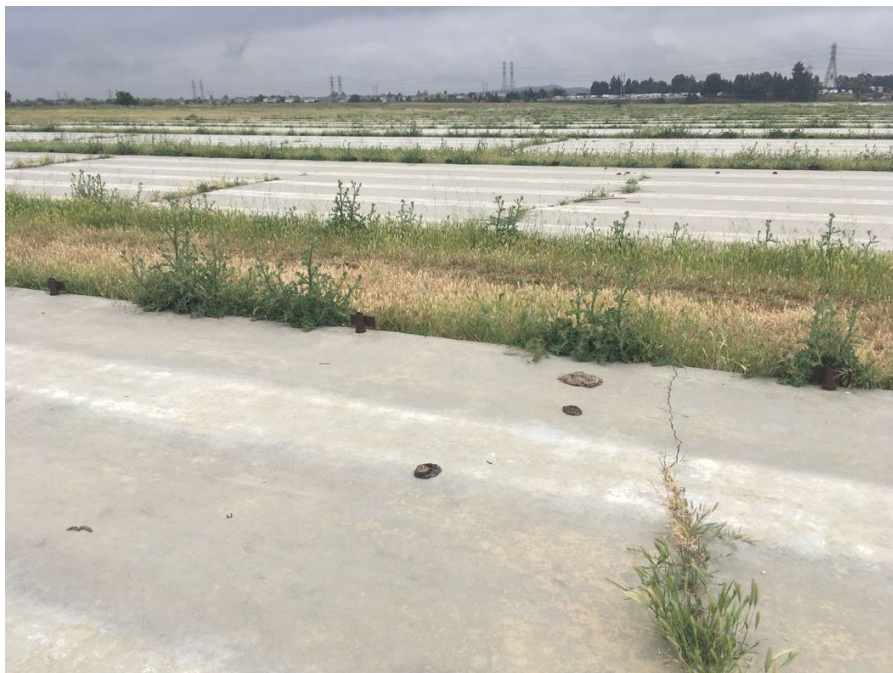
Photo 4. Picture of concrete pads within the central portion of the project, facing south.
