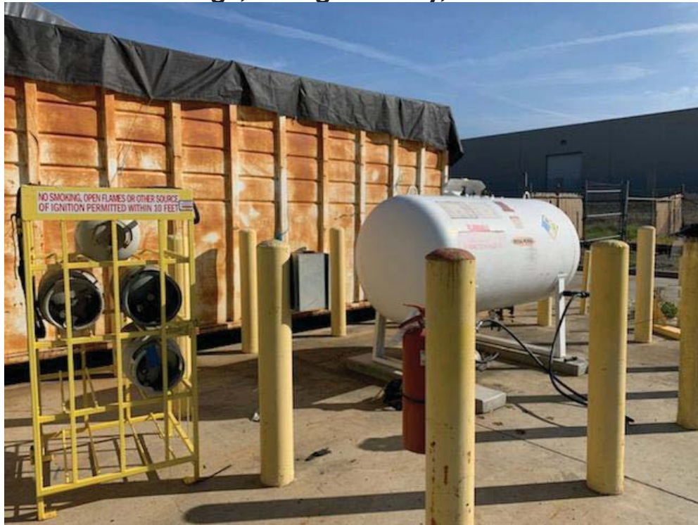
15. Showing AST filled with propane
