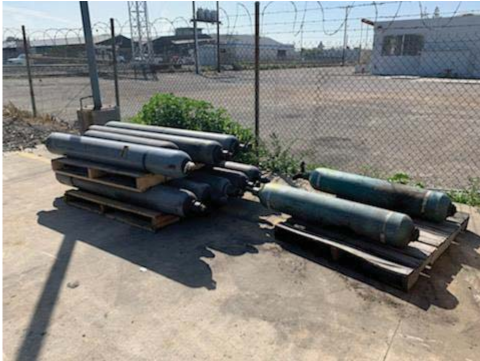
27. View of high-pressure nitrogen tanks
