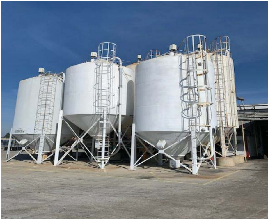
22. Containers holding plastic granules.
