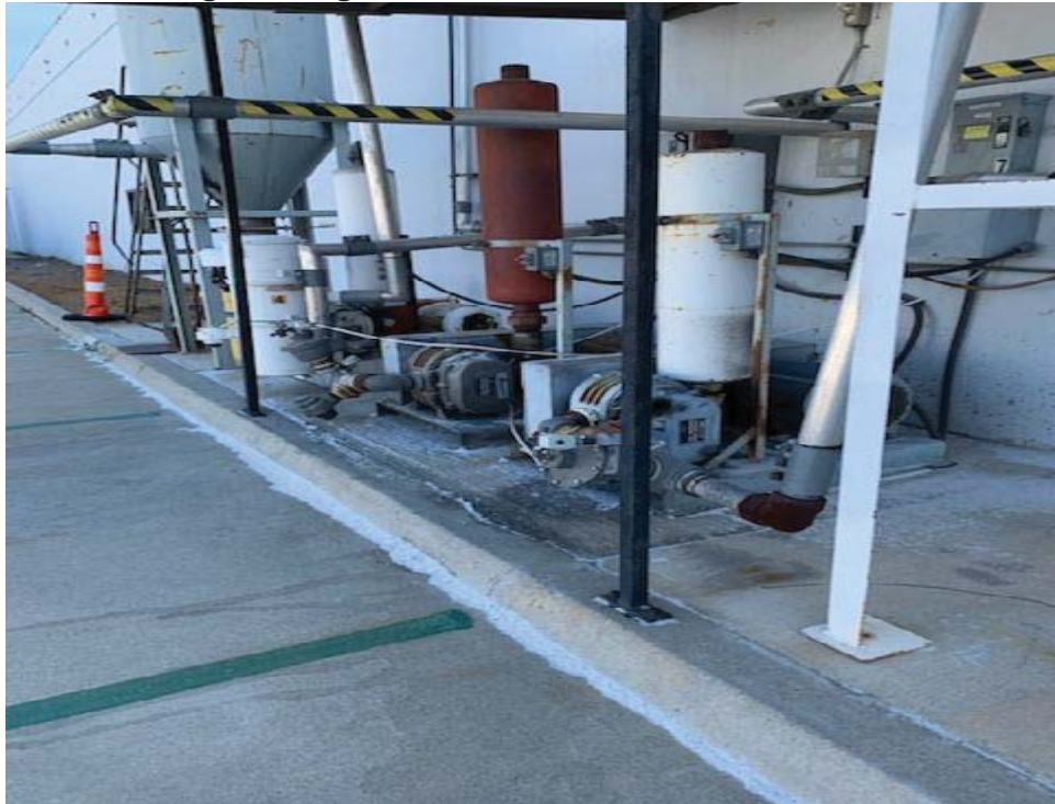
20. Showing equipment related to plastics production. Some spent plastics debris along curb and around equipment.
