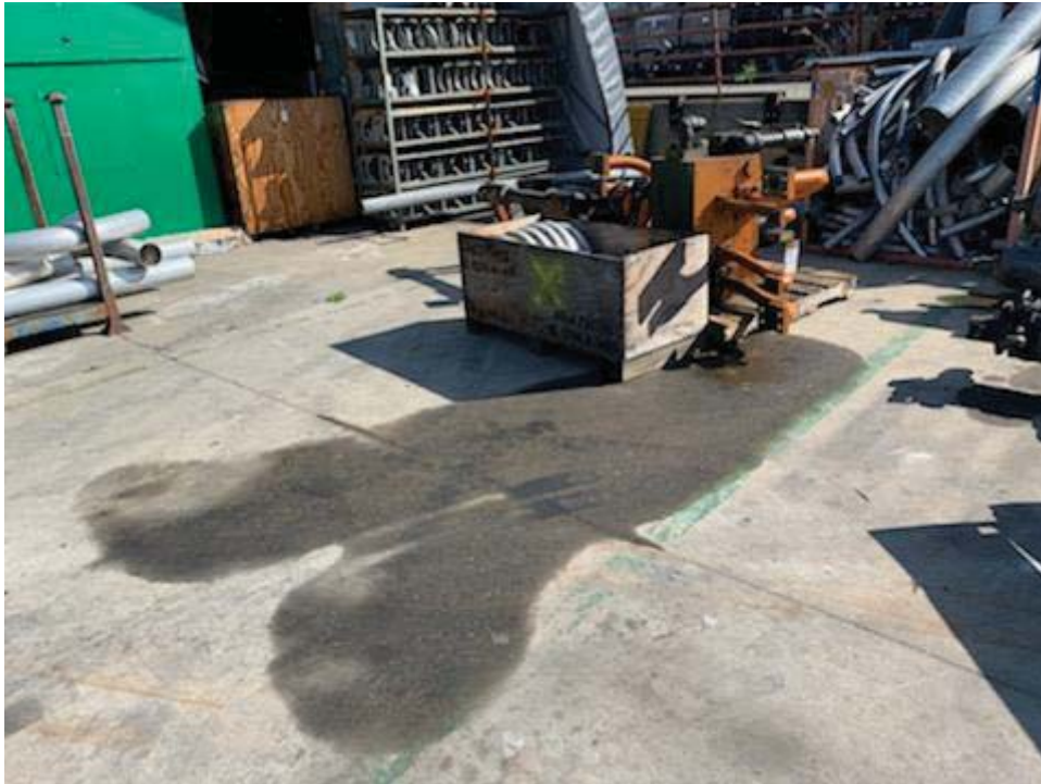
26. Showing motor oil staining on concrete.
