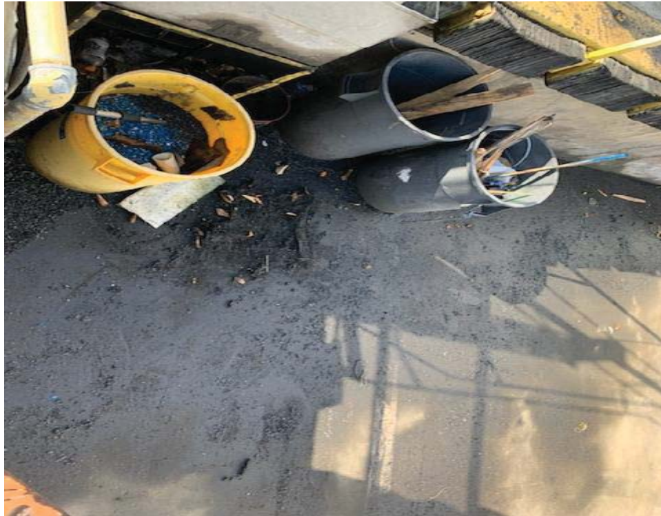
9. Showing garbage cans with some staining on the concrete.
