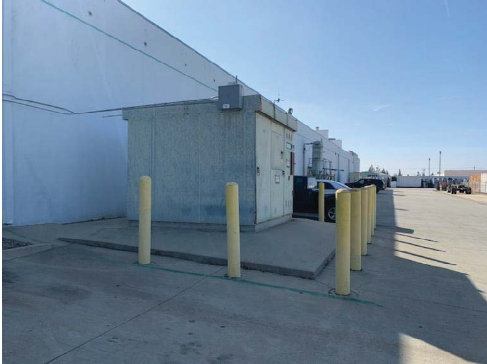
19. Showing electric generator.
