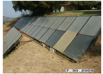
Ground-mounted solar panels
