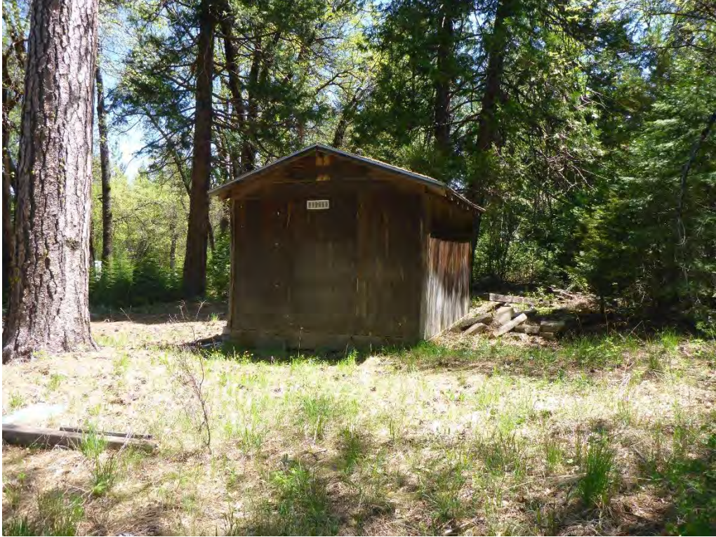
Shed behind dental clinic building, with bat guano staining near roof peak
