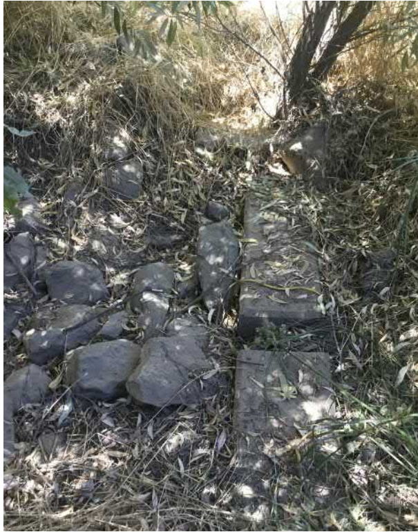
23. View of stormwater culvert and basin that drains Basin 1. This receives water from the library parking lot and the stormwater detention swale/13th street.
