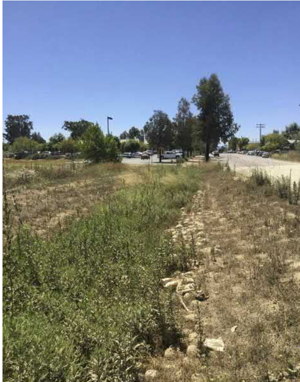
19. View of stormwater detention swale between 13th street road and Basin 1. This receives water from the paved 13th street to the south.
