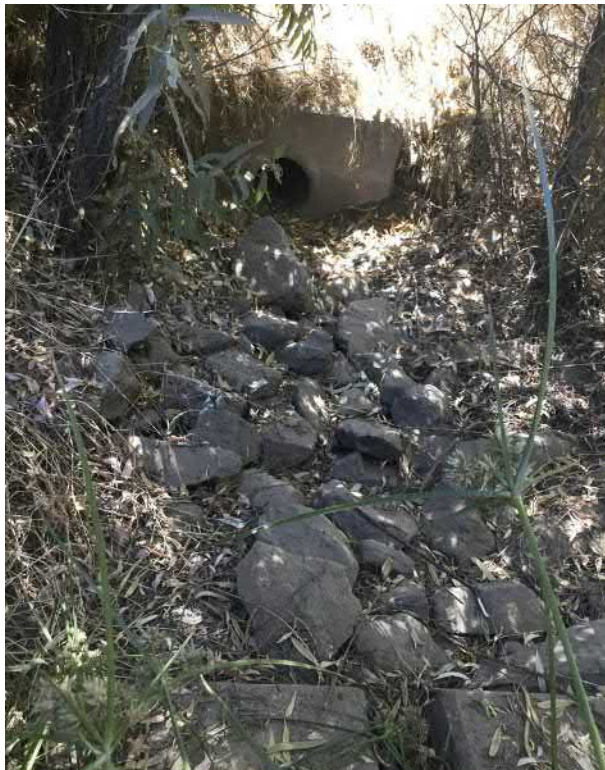
24. View of stormwater culvert and basin that drains Basin 1. This receives water from the library parking lot and the stormwater detention swale/13th street.
