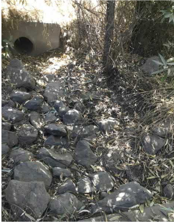
21. View of stormwater culvert and detention basin that drains Basin 1. This receives water from the library parking lot and the stormwater detention swale/13th street.
