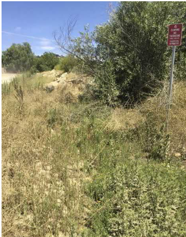
20. View of stormwater detention swale between 13th street road and Basin 1. This receives water from the paved 13th street to the south.
