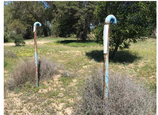
Photograph 6. View of two vent pipes located in the southwestern corner of the subject property.
