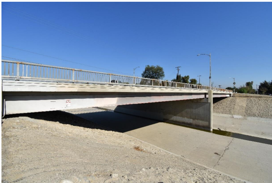
Figure 17 White Oak Avenue Bridge-Photograph Taken from the East on the South Bank of the River; Northwest-facing
