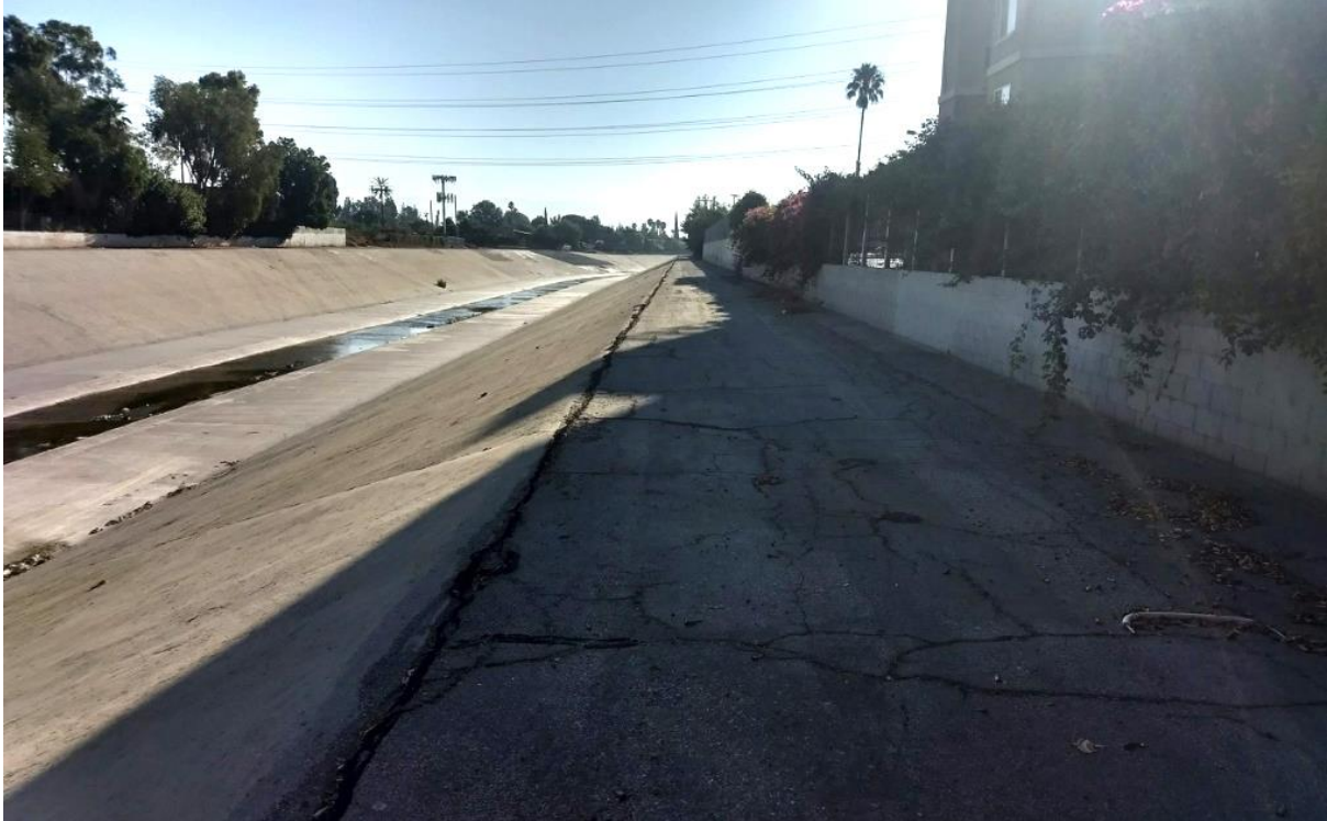
Photograph 5. View of concrete lined portion of the Los Angeles River on the far western end of the Study Area. Photo facing northeast.
