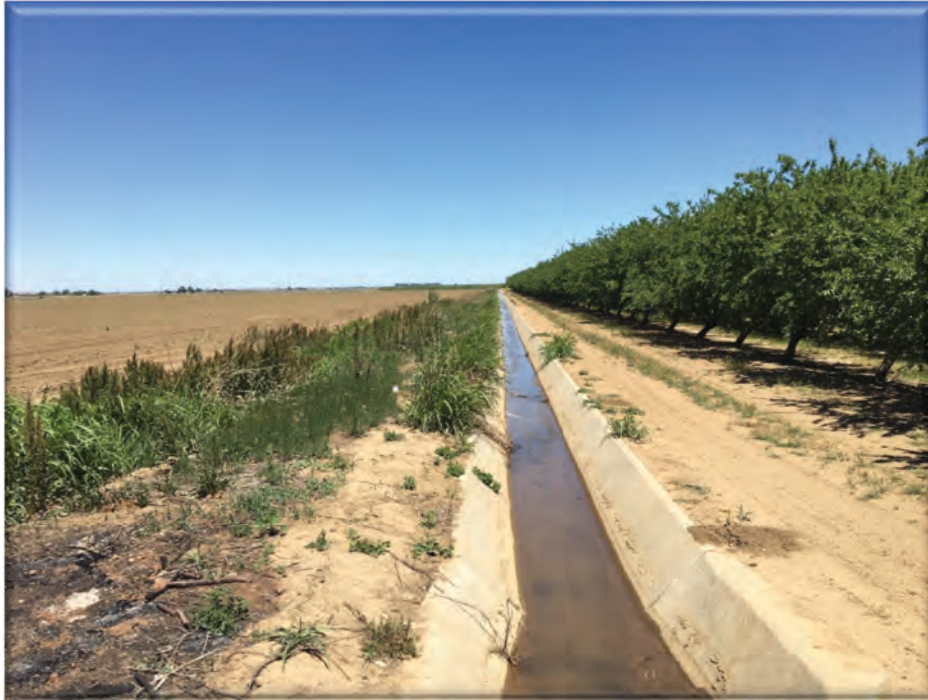
Plate 6. Looking north along the irrigation canal bordering the eastern boundary of the project. This is also a concrete-lined permanent water conveyance feature.
