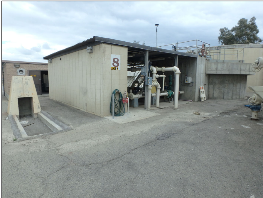
Figure 11. Overview of Building 8 (DAFT/ WS Pump Station), and DAFT/ WS Tank (1972), looking southeast.
