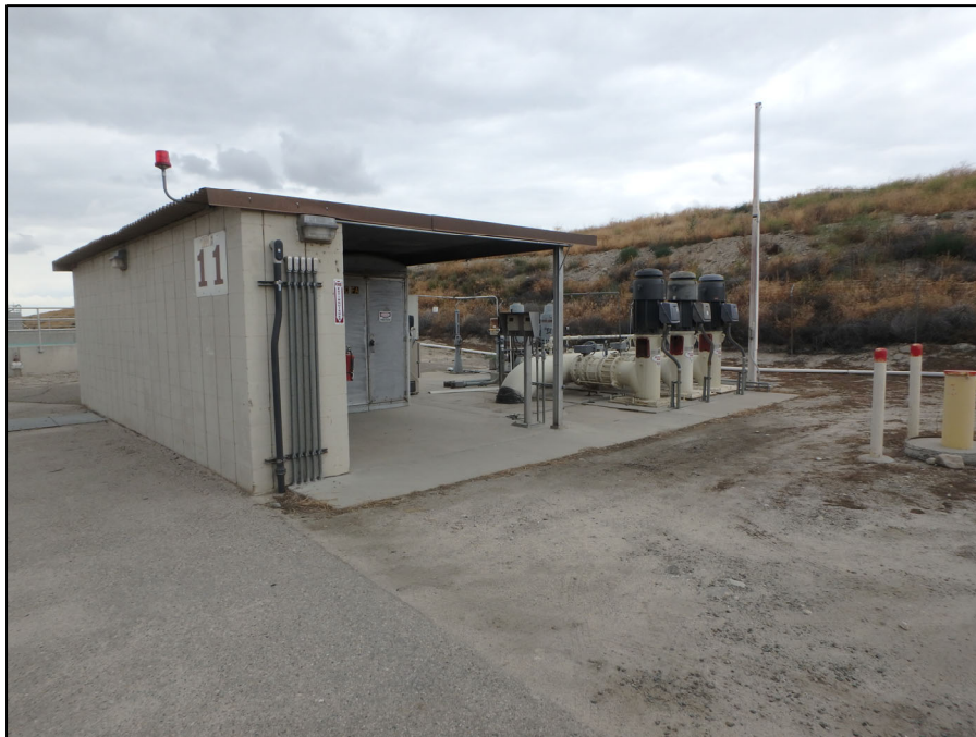
Figure 9. Overview of Building 11 (Stand-by Power Facility) and the Final Effluent Pump Station (1972), looking northwest.
