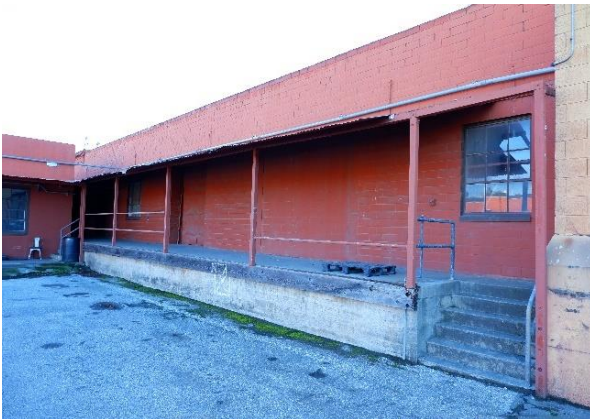
Figure 33. Loading dock on the north side of the 1931 warehouse, extending into the 1125 Arguello Street parcel, looking southeast.
