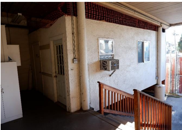
Figure 37. Enclosed room addition at the north end of the loading dock structure, looking southeast.
