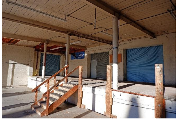
Figure 36. Concrete loading dock with rollup doors from the adjacent 1980 warehouse-office building (left) and the 1931 warehouse (center and right).
