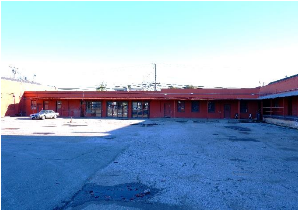
Figure 26. Rear (west) façade of the 1931 office building (left) and 1959 office building addition (right), looking east.
