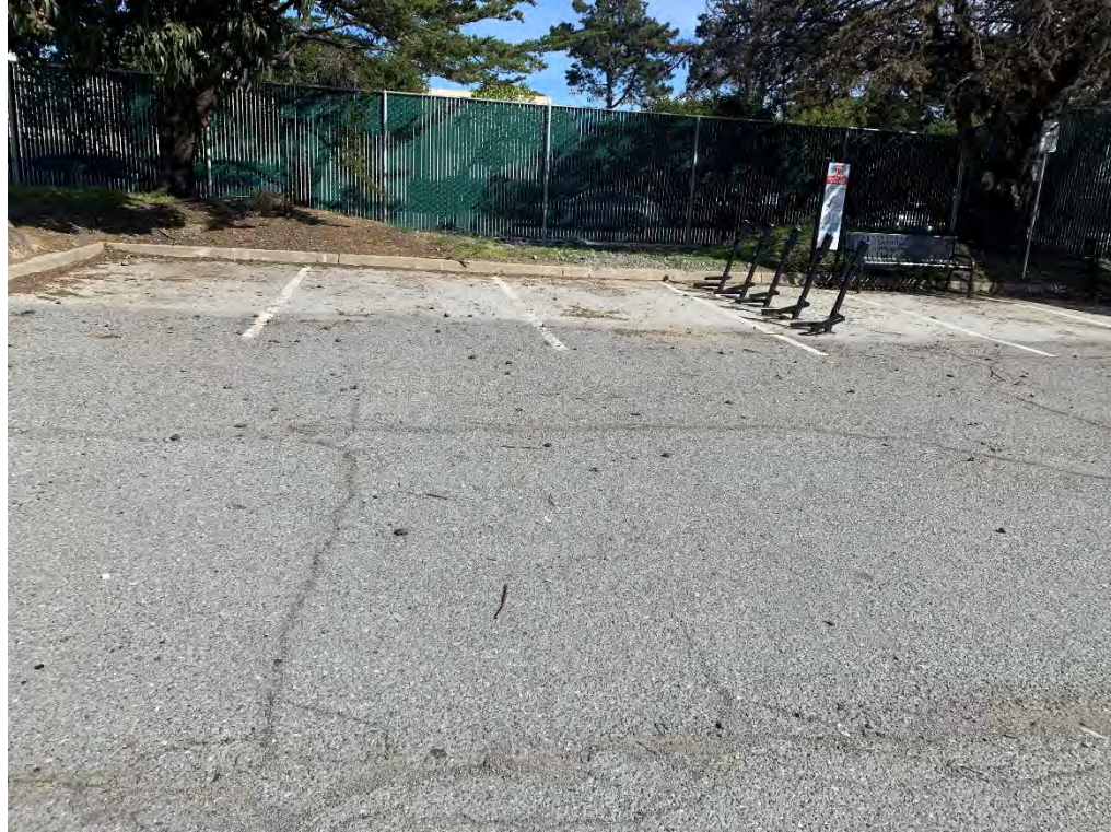
Parking area at northern edge of Target Site, looking north toward Newhall Street
