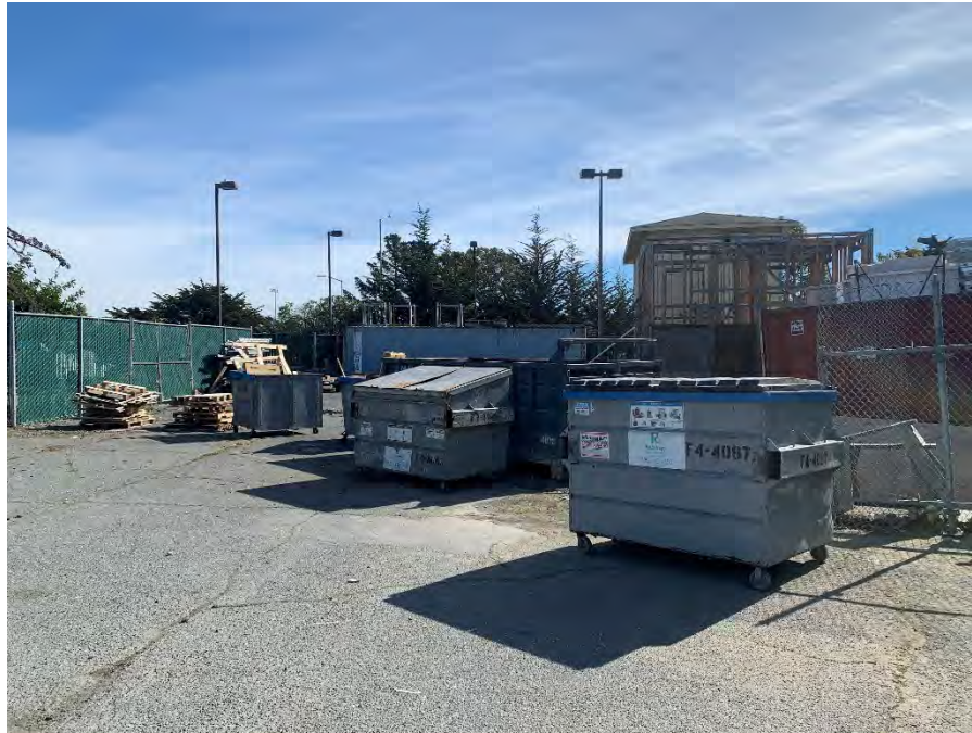
Looking east at storage and construction instruction area at north portion of Target Site.
