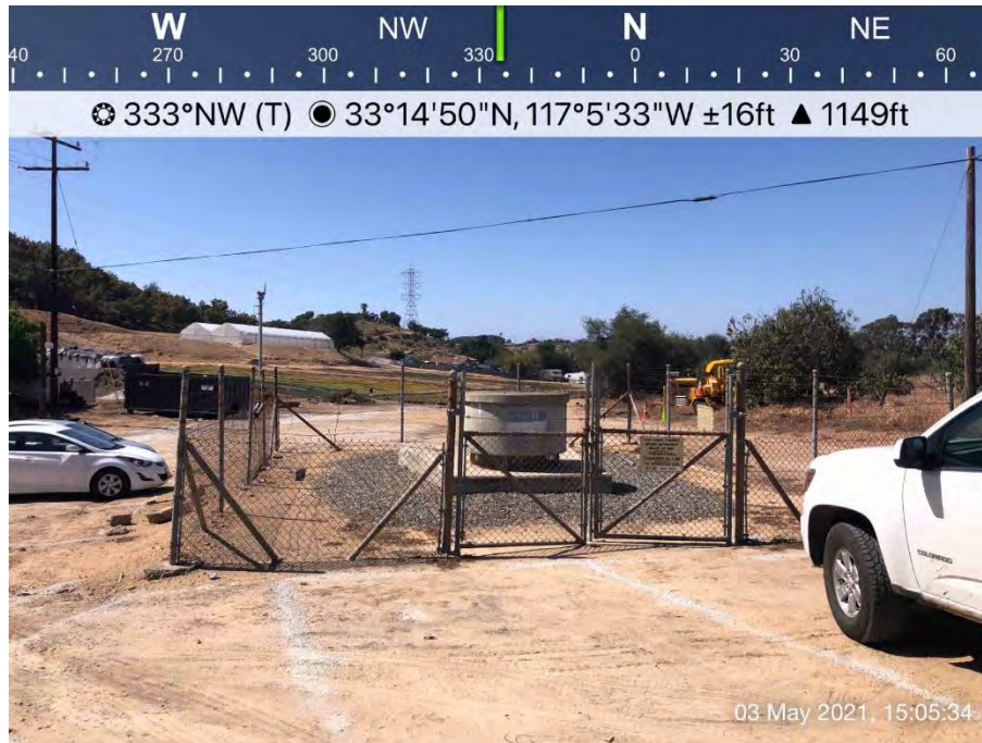
Photo 7: The potential work area within Study Area 2 is centered around the upstream Red Mountain Tunnel bifurcation structure. The structure is surrounded by bare ground, non-native grassland and intensive agriculture (a nursery). Non-native grassland with a few oak and avocado trees falls within the potential work area east of the bifurcation structure.
