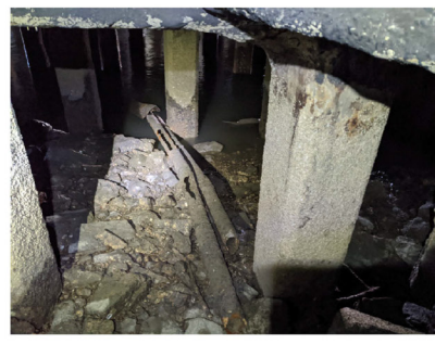
PHOTO 122 (P39_N_120119.jpg) Approxim a tely 50 ft 2 of exposed fill.
