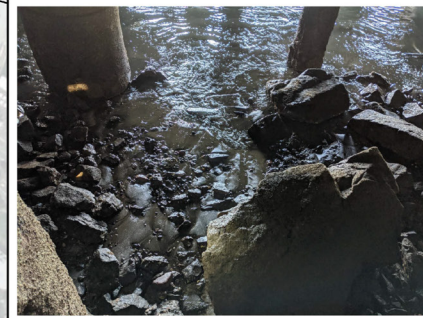
PHOTO 145 (AQ_N_F2.jpg) Approxim a tely 50 ft 2 of exposed sedim ent.
