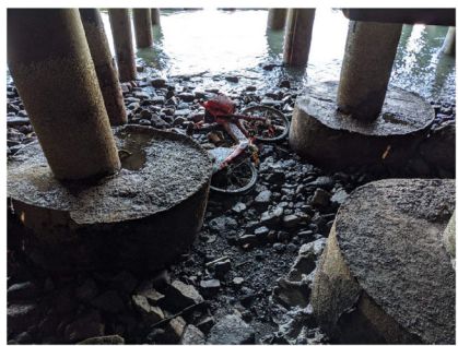
PHOTO 48 (P435_N_8281.jpg) Approxim a tely 25 ft 2 of exposed fill.
