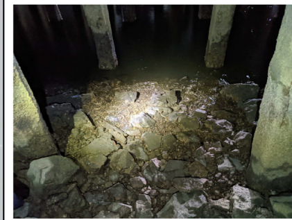
PHOTO 123 (P39_N_126124.jpg) Approxim a tely 75 ft 2 of exposed fill.
