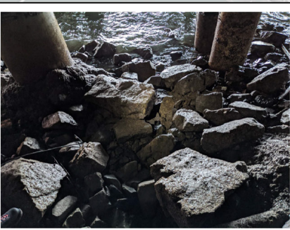
PHOTO 14 (P44_N_7980.jpg) Approxim a tely 10 ft 2 of exposed fill.
