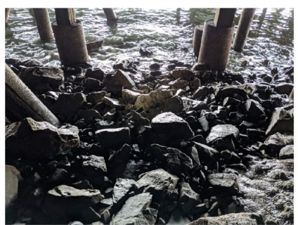
PHOTO 18 (P44_N_7576.jpg) Approxim a tely 10 ft 2 of exposed fill.
