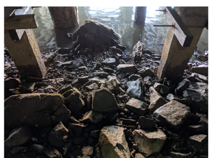
PHOTO 95 (P41_N_115116.jpg) Approxim a tely 50 ft 2 of revetm ent la cking la rge rock.
