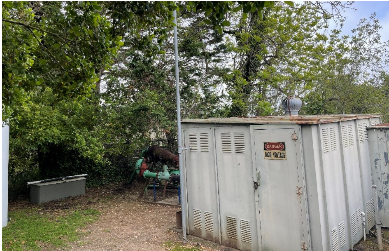
Photograph 5. The northeast side of the study area, showing the existing Country Club well pump enclosure.
