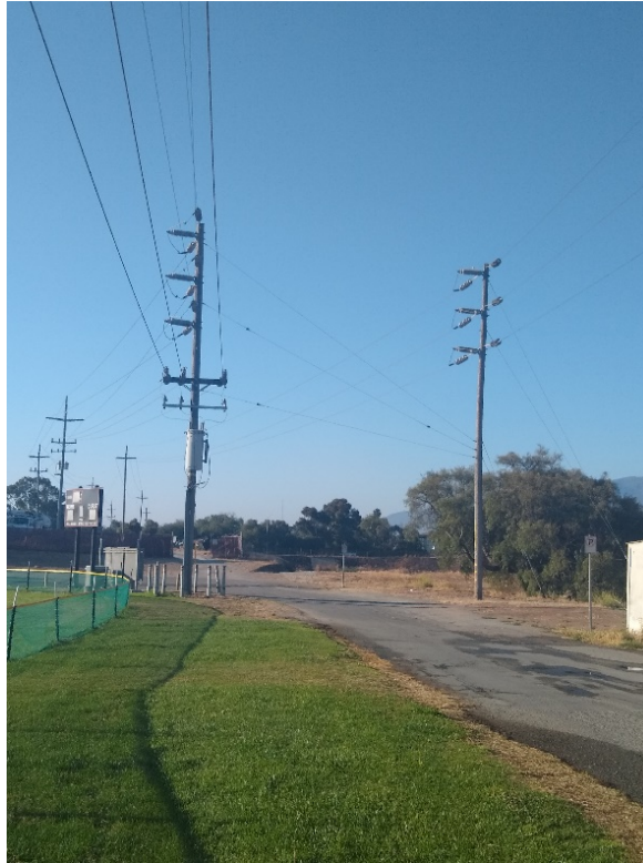
FIGURE 9: CAISO/PG&E POWER LINES (69 KV EACH) IN CENTENNIAL PARK
