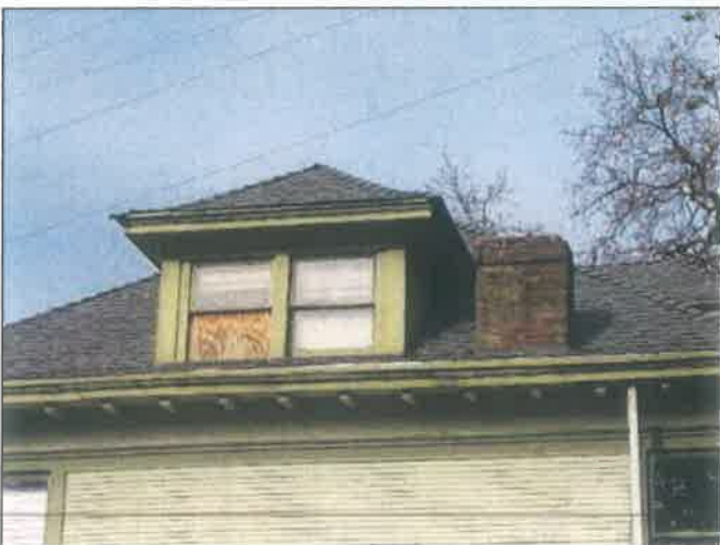
65. Asphalt shingle roofing at the residential building. Note boarded up window.
