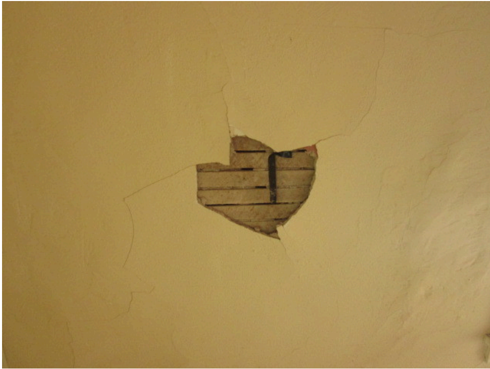
33. Damaged wall plaster at the house
