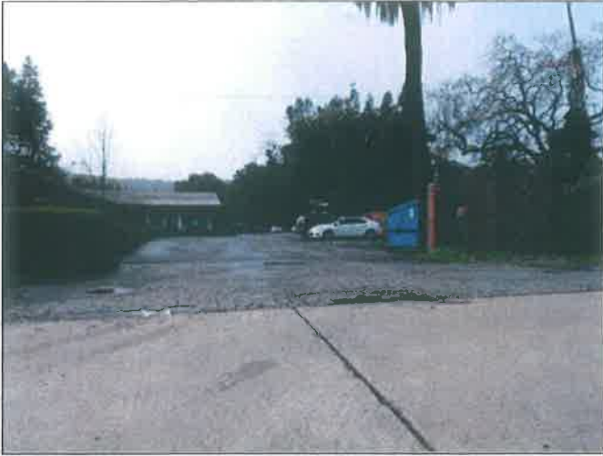
1. Property entrance drive lane. Note pothole and alligator asphalt.
