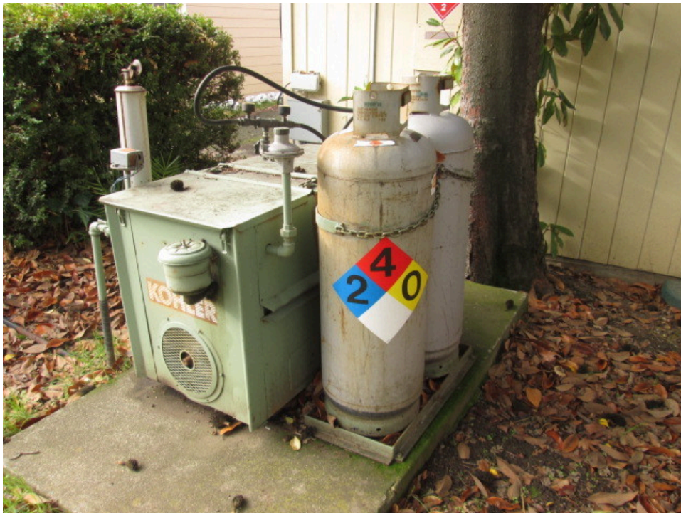
24. Natural gas powered electrical generator and propane storage tanks
