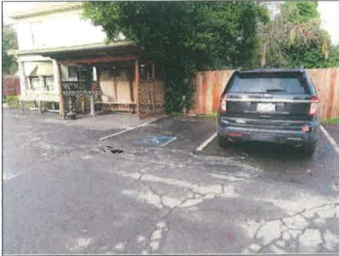
9. ADA-designated parking stall and cracked asphalt pavement
