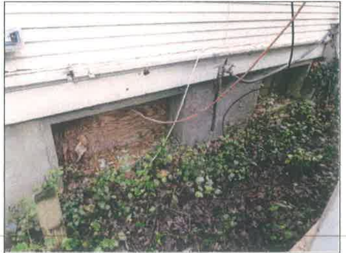
54. Broken window covered with plywood at the residential building basement
