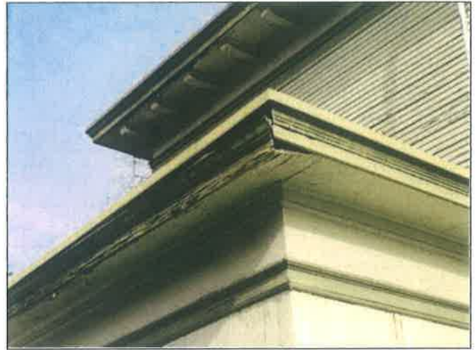
46. Dry rot at residential building eaves
