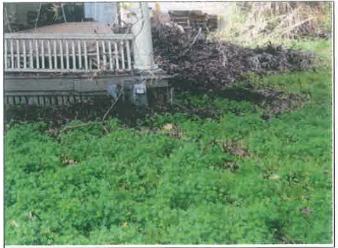
26. Natural gas meter at the residential building
