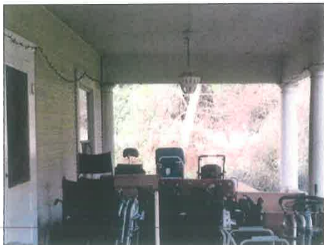
23. Porch lighting fixture at the residential building
