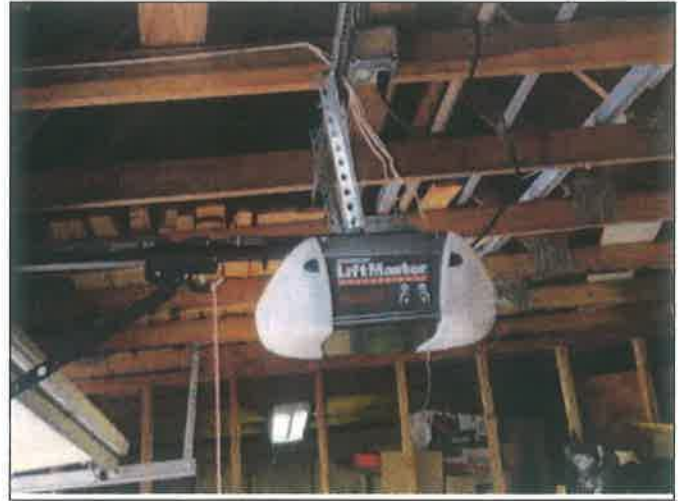
58. Automatic garage door operating mechanism
