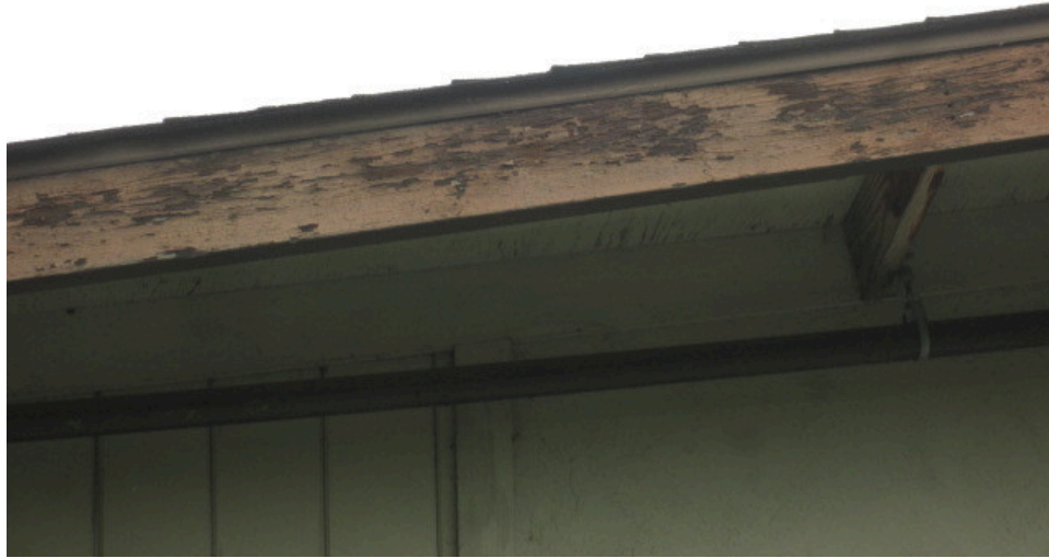
19. Flaking paint on the convalescent home
