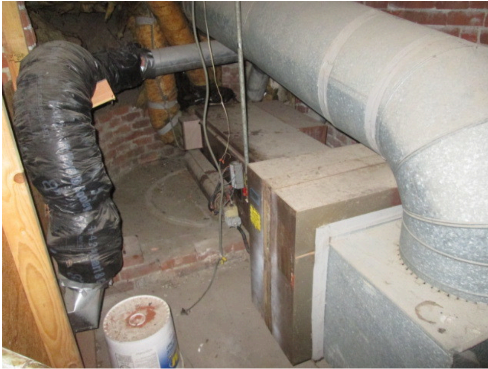
35. Furnace unit in the basement
