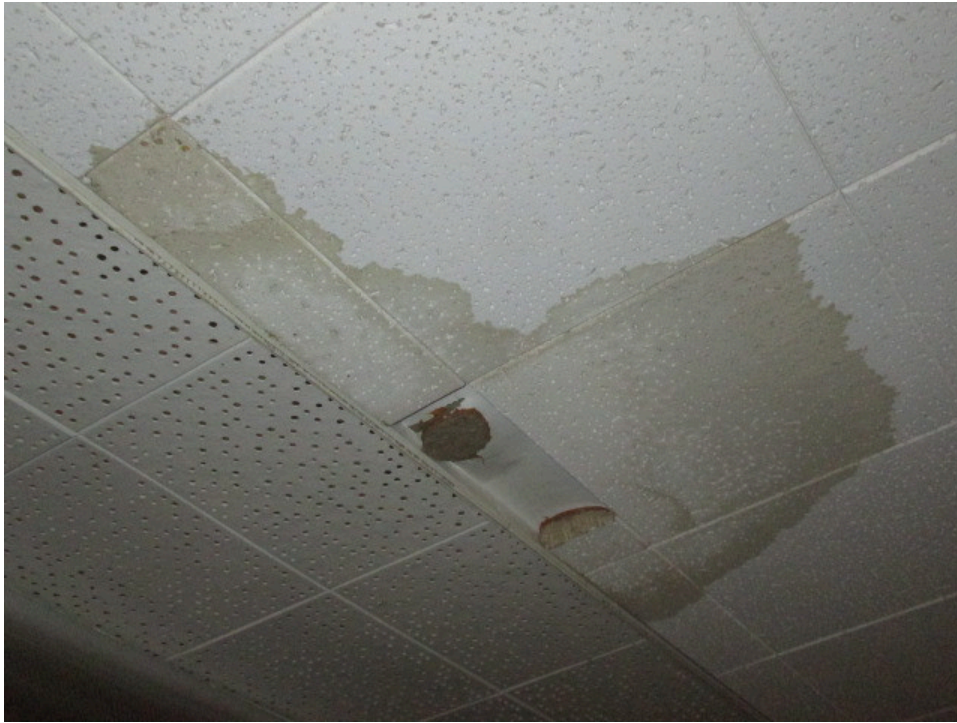
17. Stained ceiling tiles at the convalescent home
