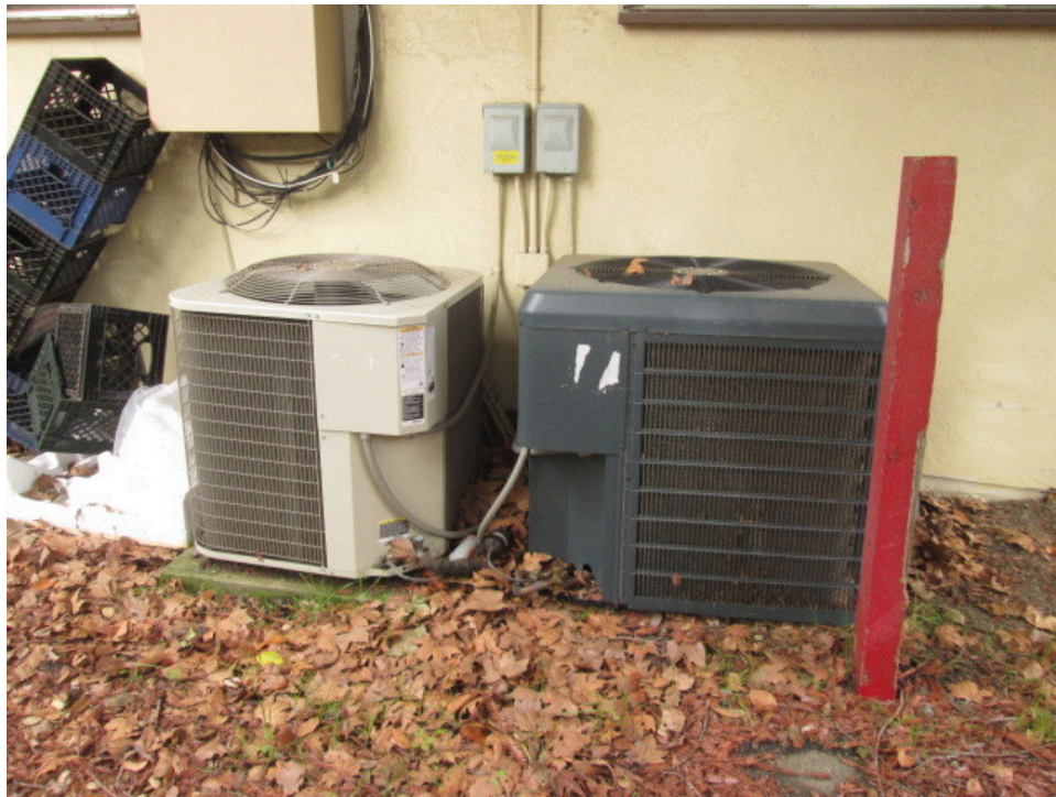
20. Split system condensing units at the convalescent home
