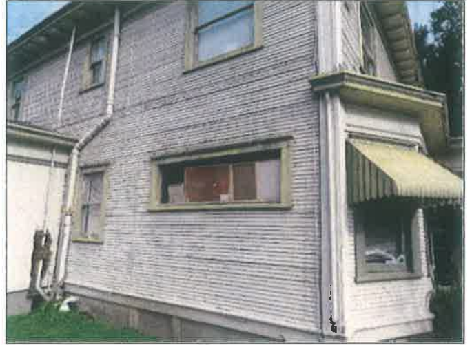
52. Windows at the residential building. Note boarded up window
