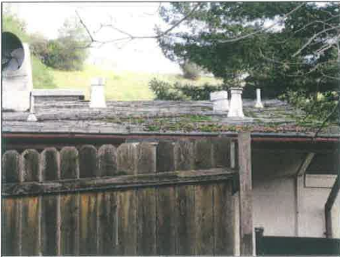
63. North portion of the convalescent building roof showing moss buildup
