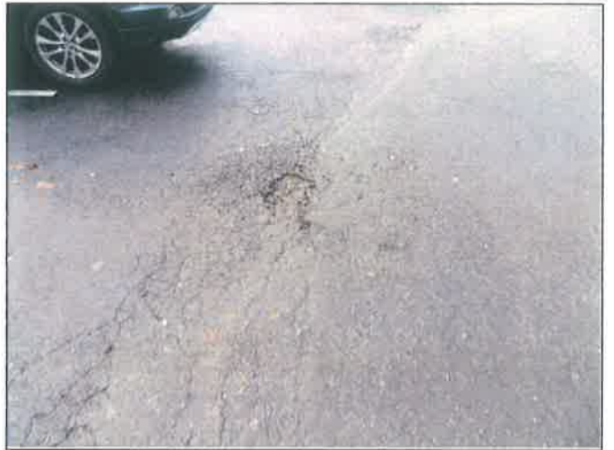
4. Deteriorated asphalt pavement
