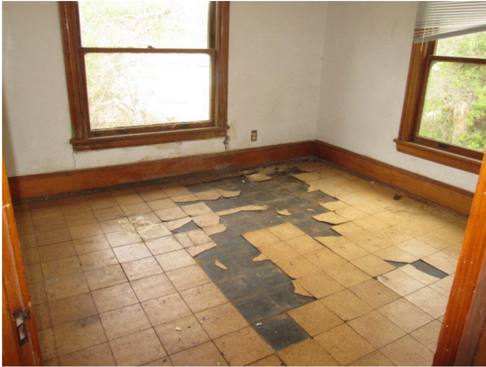
31. Damaged floor tiles in a bedroom at the house
