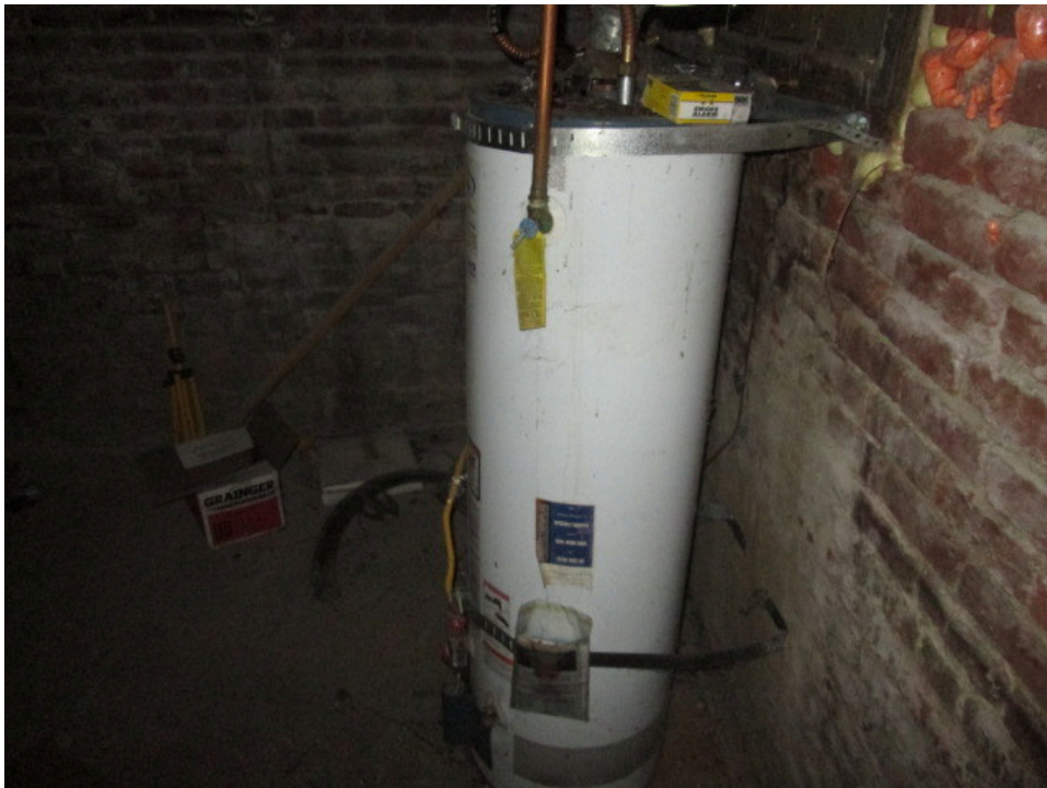
36. Water heater for the house
