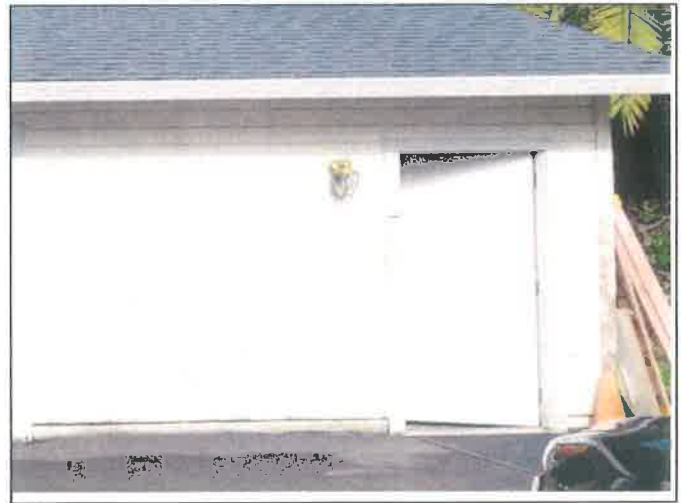
22. Building-mounted light fixture at the garage building
