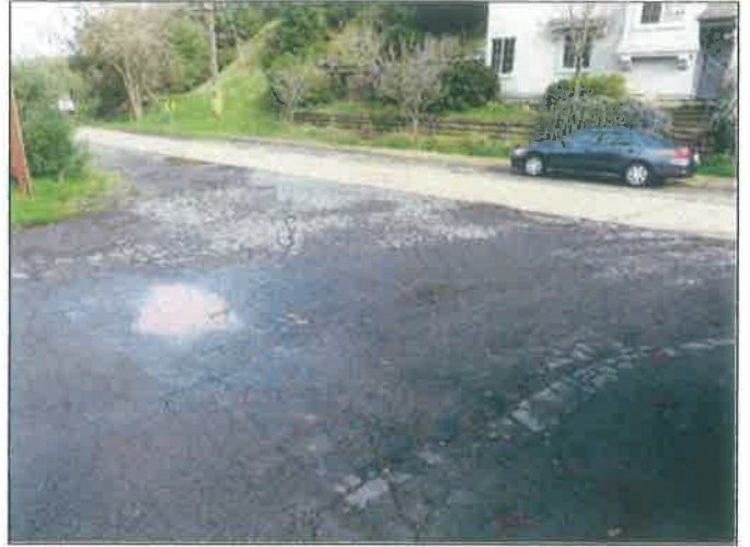
2. Close-up view of damaged asphalt pavement
