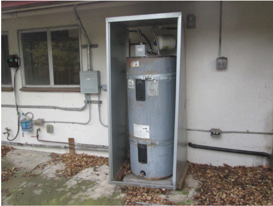
21. Water heater for the convalescent home
