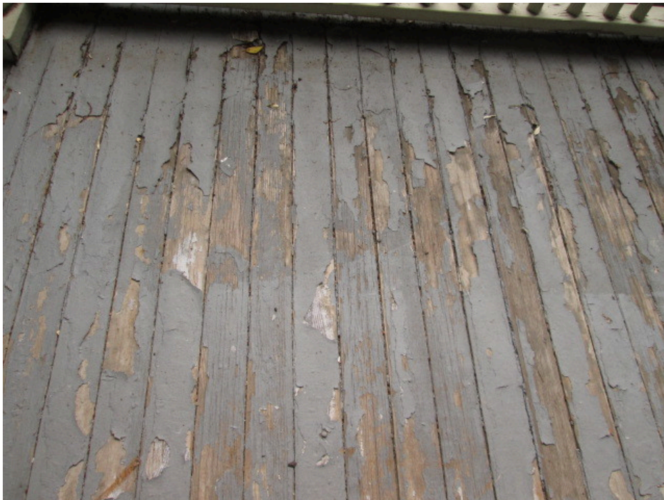
38. Flaking exterior paint at the house
