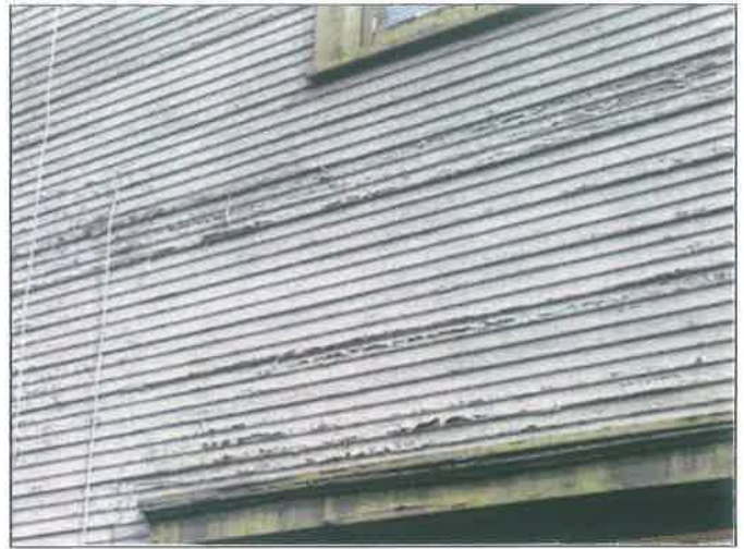
44. Deteriorated paint finish at the residential building
