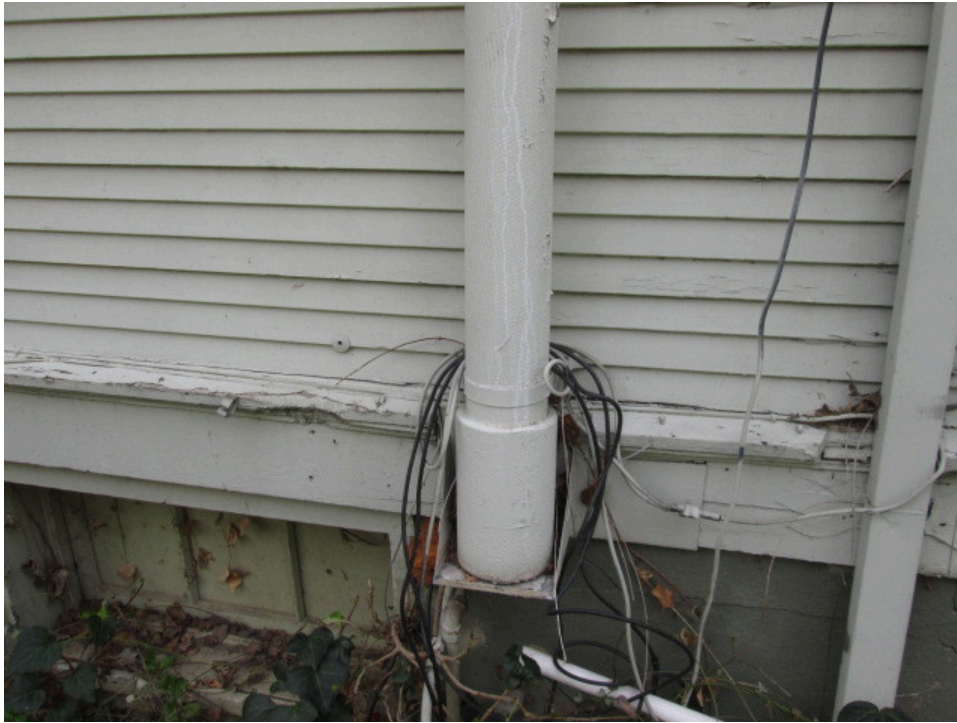
37. Suspect asbestos containing cement vent pipe
