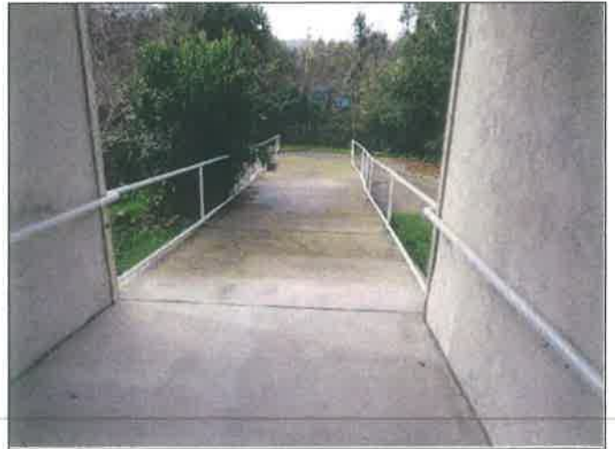
12. Ramp and guardrails at the west side of the convalescent hospital building
