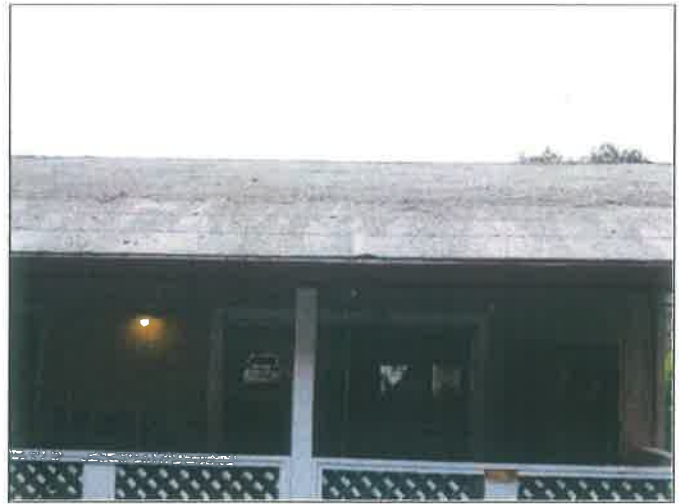
62. Roof showing missing loose-laid aggregate
