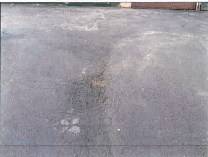
5. Deteriorated asphalt at the west parking area drive lane
