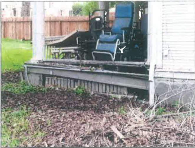
49. Dry rot at the porch framing of the residential building
