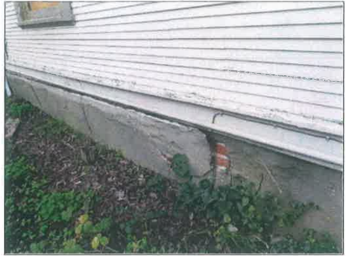
50. Delaminated stucco at the lower portion of the residential building north wall
