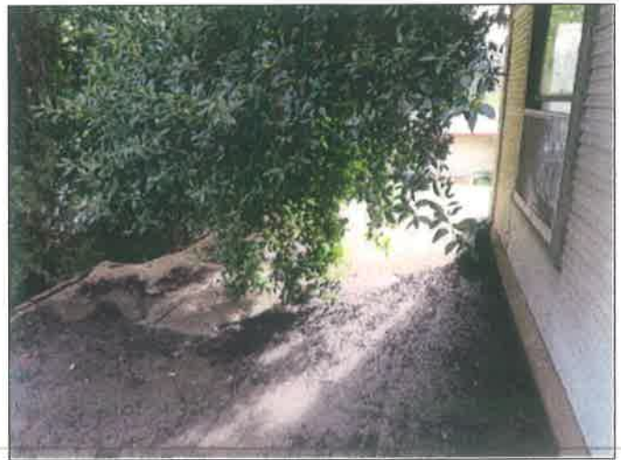
18. Tree overhanging touching the porch at the residential building
