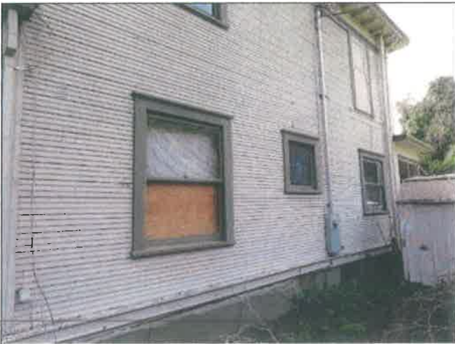
53. Boarded up window at the north side of the residential building
