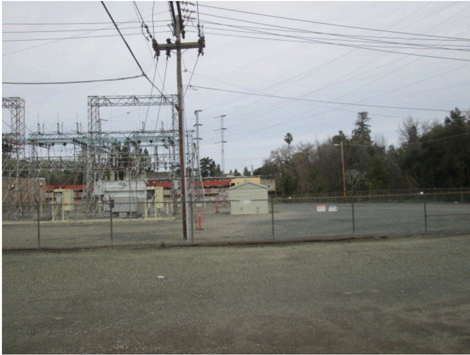
51. Electrical substation on the adjacent property to the northwest
