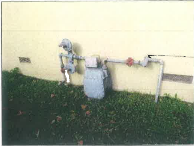
25. Natural gas meter at the convalescent hospital building
