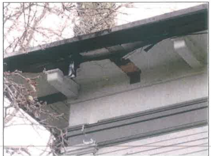
48. Dry rot at the porch canopy at the residential building
