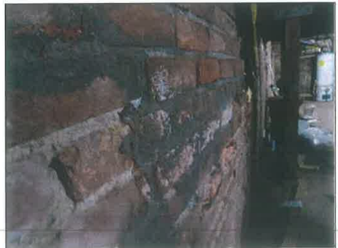
30. Brick masonry perimeter wall showing bowing at the residential building
