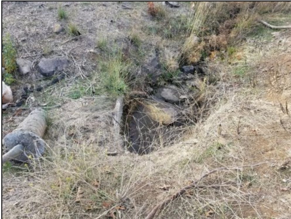
7 : View of the drainage outflow on the central portion of the site.
