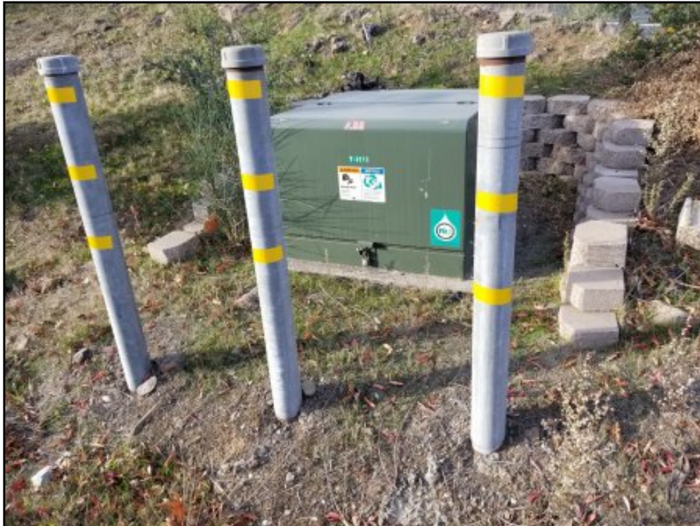
9 : View of the on-site pad mounted transformer on the northwestern portion of the site.
