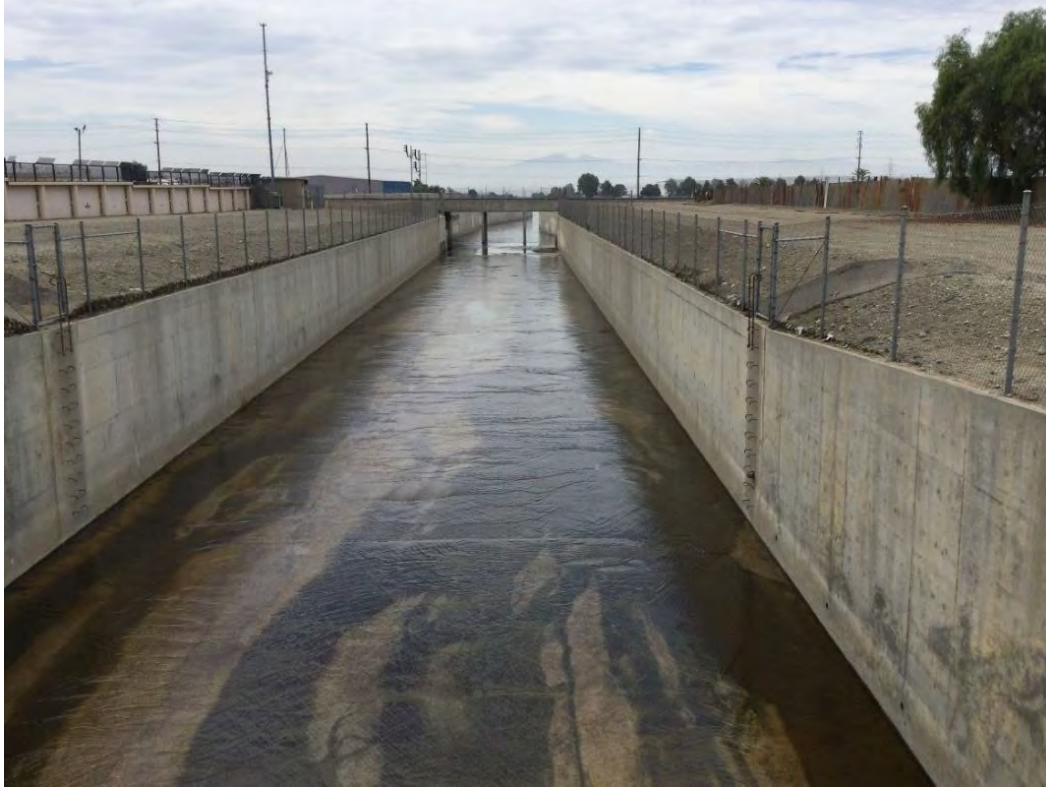
Figure 5-12. Overview of San Sevaine Channel at intersection of Hickory and Whittram avenues (BNSF Railroad crossing in background), facing south.
