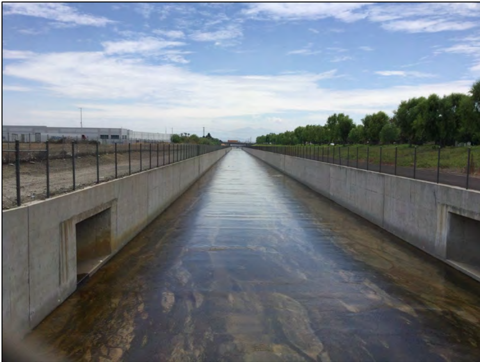
Photograph 4. Overview of San Sevaine Channel at intersection of Commerce Drive and San Bernardino Avenue (Point 4) with Valley Boulevard overcrossing in background, facing south, July 26, 2021.
