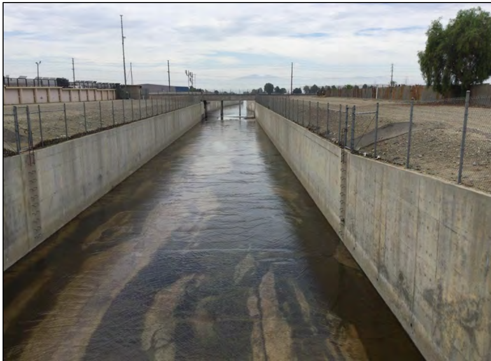
Photograph 2. Overview of San Sevaine Channel at intersection of Hickory and Whittram avenues (Point 2) with BNSF Railroad overcrossing in background, facing south, July 26, 2021.
