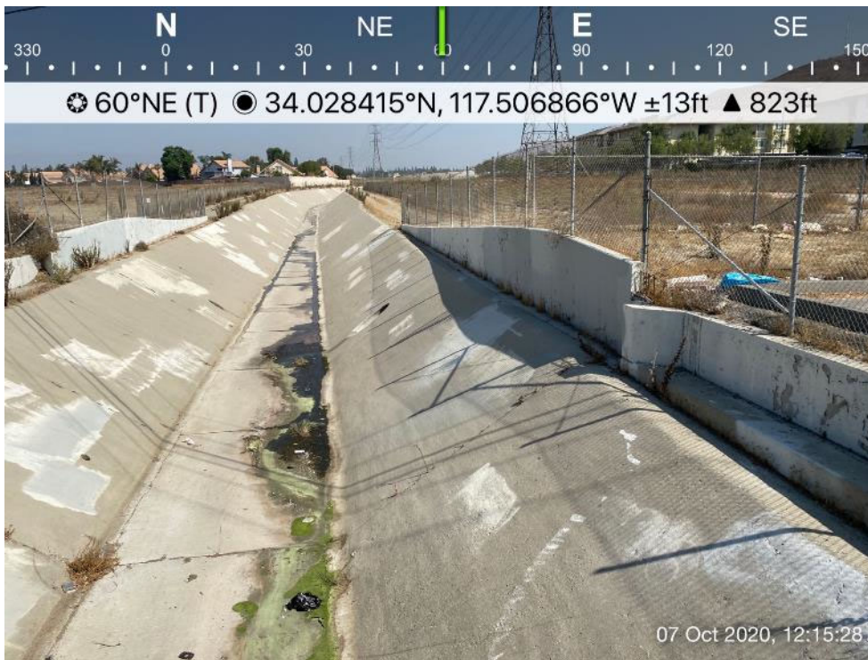
Photo 6. View of concrete Drainage looking downstream Country Village Road north of SR 60.
