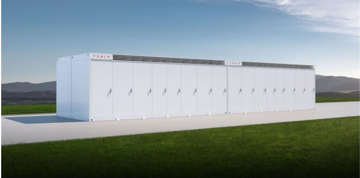
Photo PD-3: Modular Battery Structure for Energy Storage
