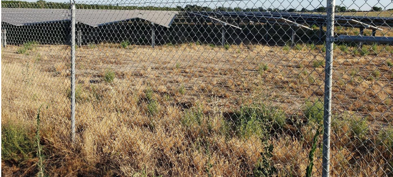
Photo PD-1: Typical Single-Axis Solar Array and Chain Link Fence
