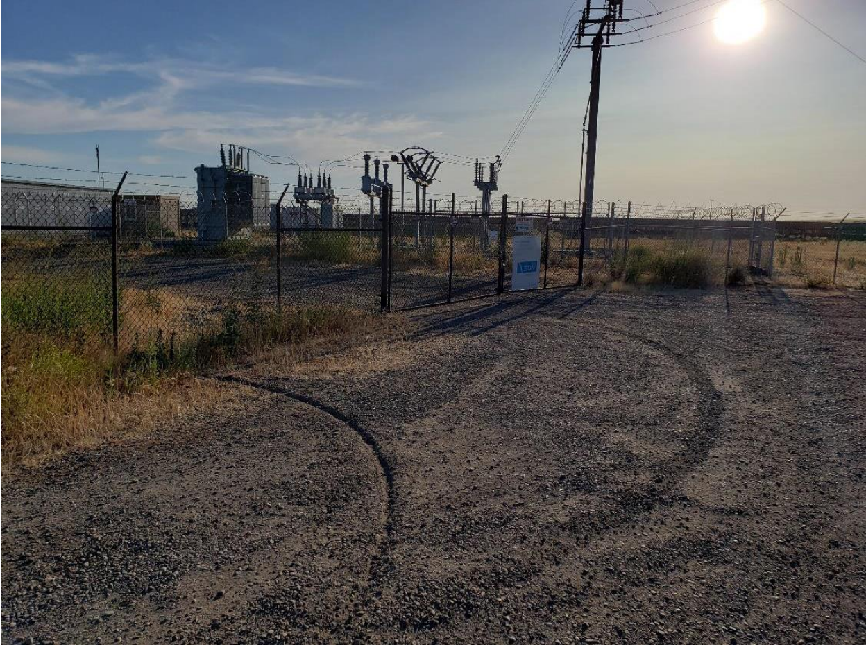
Photo PD-2: Typical Substation Facilities
