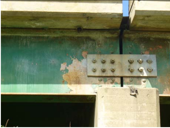
Photo 7: Detailed view of paint chipping on bridge substructure.
