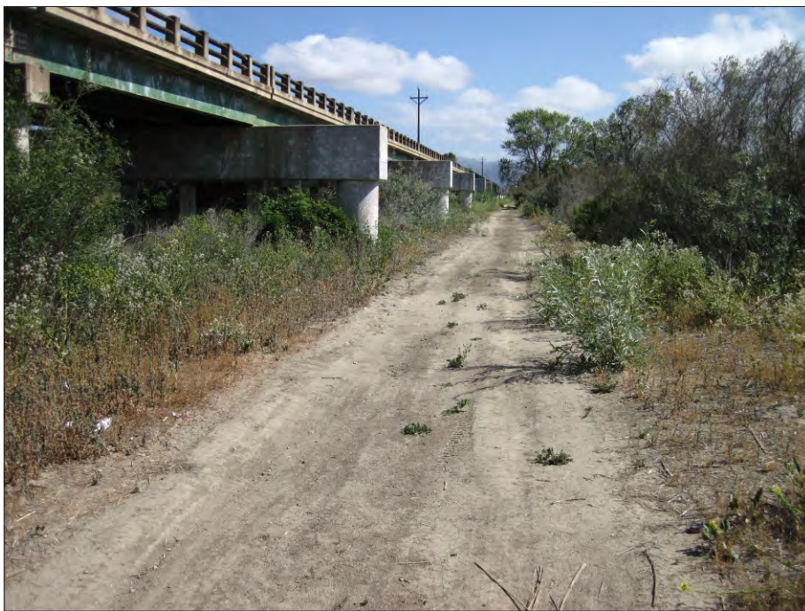
Figure 8b: Salinas River floodplain (high flow channel), access road and Gonzales River Road Bridge, willow and mulefat along road and Fremont cottonwood in right background, view from upstream of the bridge to the northeast. May 12, 2015.
