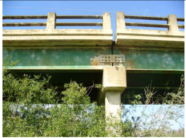
Photo 8: View of paint chipping on bridge substructure.
