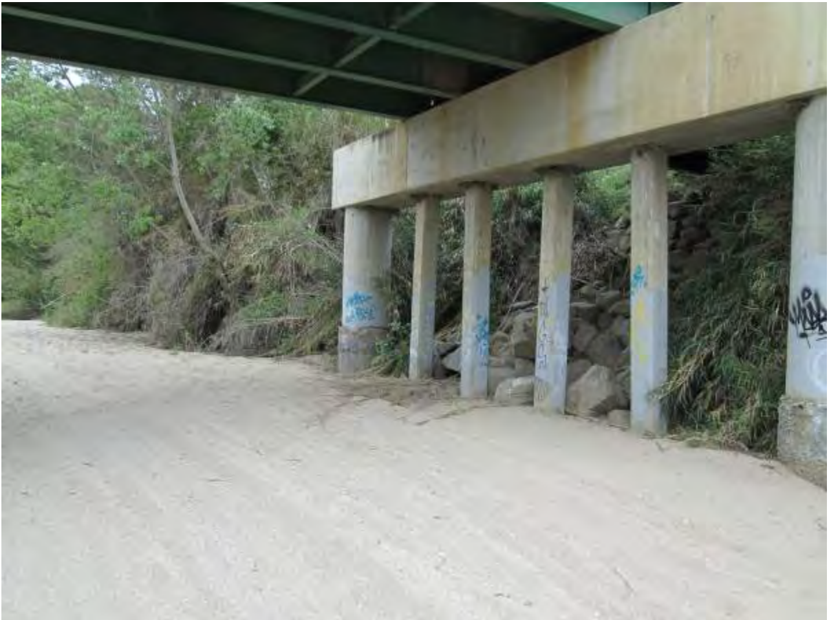
Photo 1: View of the north end of the Gonzales River Road Bridge from the Salinas River bed.
