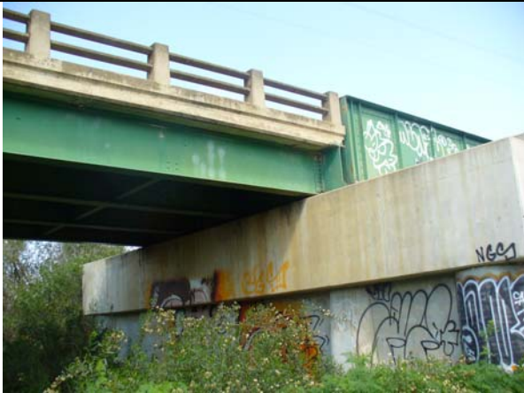
Photo 5: View of bridge substructure and abutment approximately midway along bridge where guardrails change.
