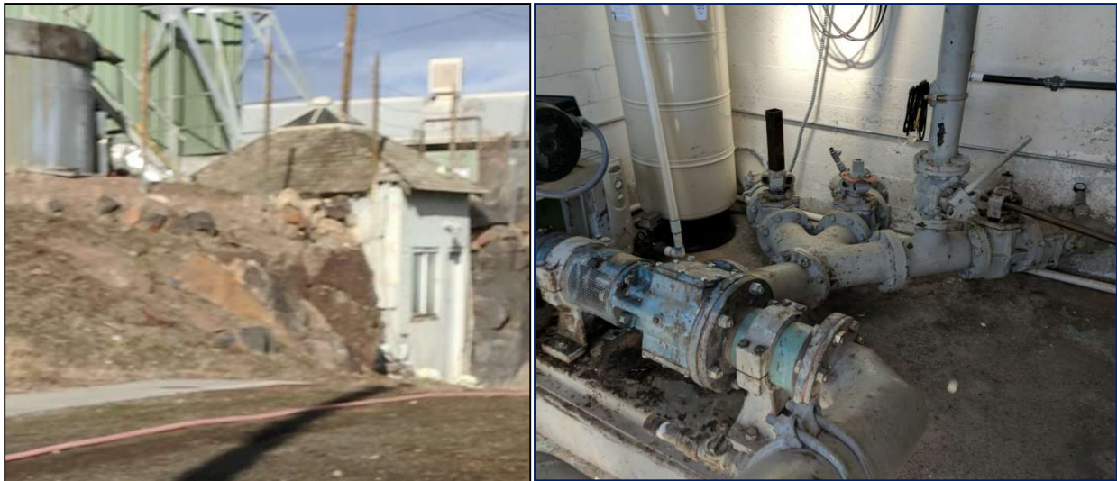
Figure 15. Sludge pump station and piping gallery.
