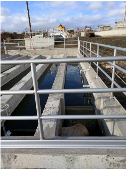
Figure 19. Chlorine contact chamber. Chlorine injection occurs in the upper structure in the background and dechlorination (sulfur dioxide injection) occurs at the chamber outfall in the foreground.
