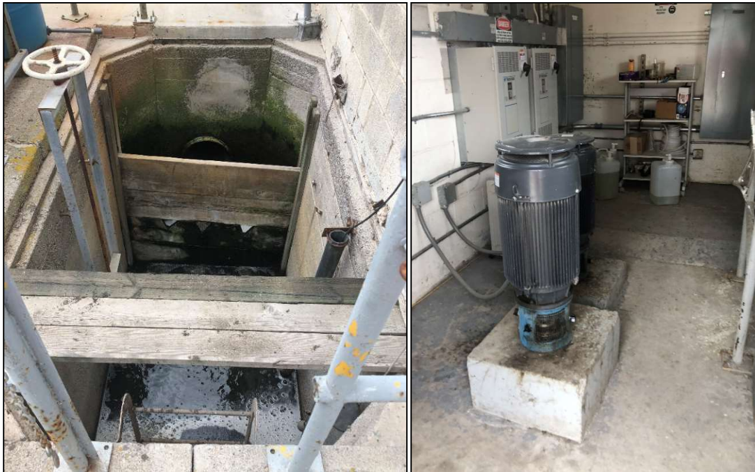
Figure 12. Recirculation flow control structure (left) and pump station to secondary clarifier (right).
