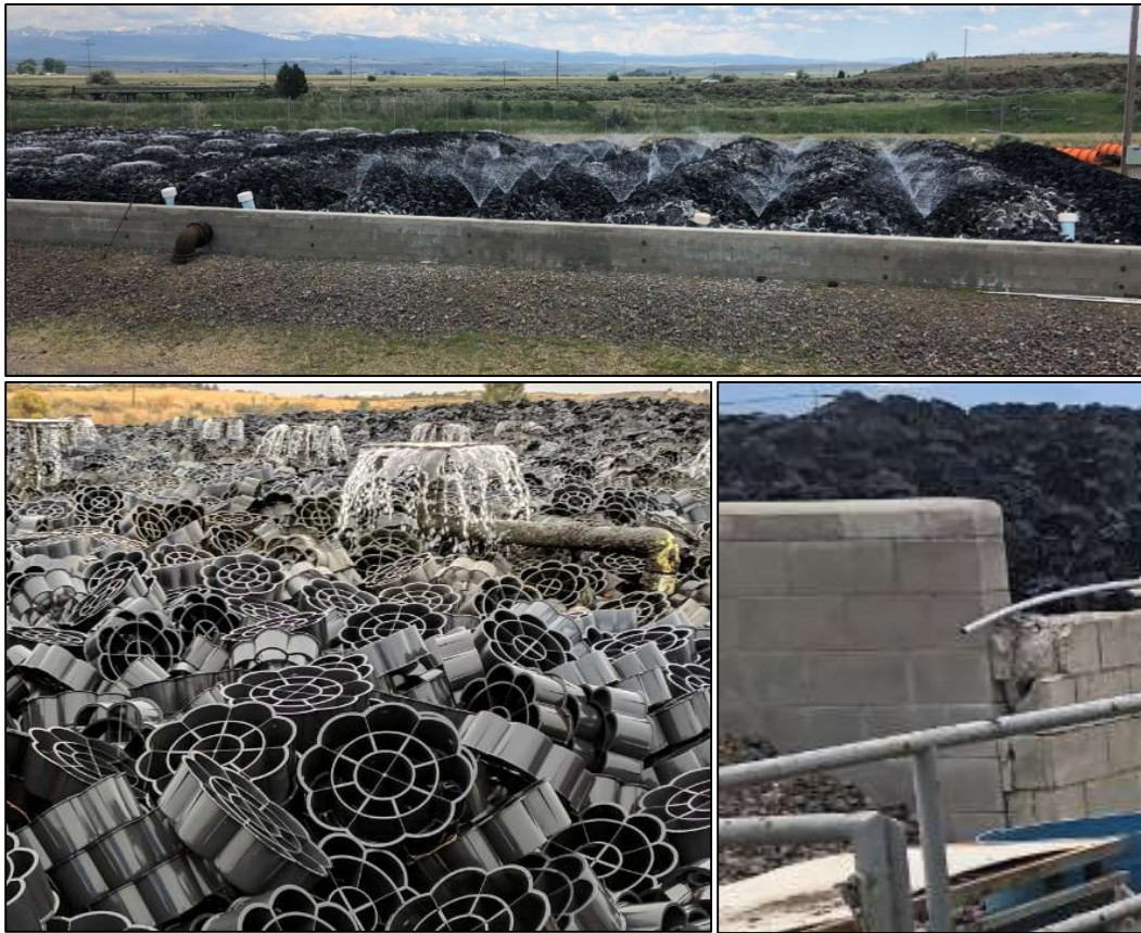
Figure 11. Trickling Filter (top) showing media (bottom left) and exterior wall where cracking has occurred in the CMU block wall (bottom right).
