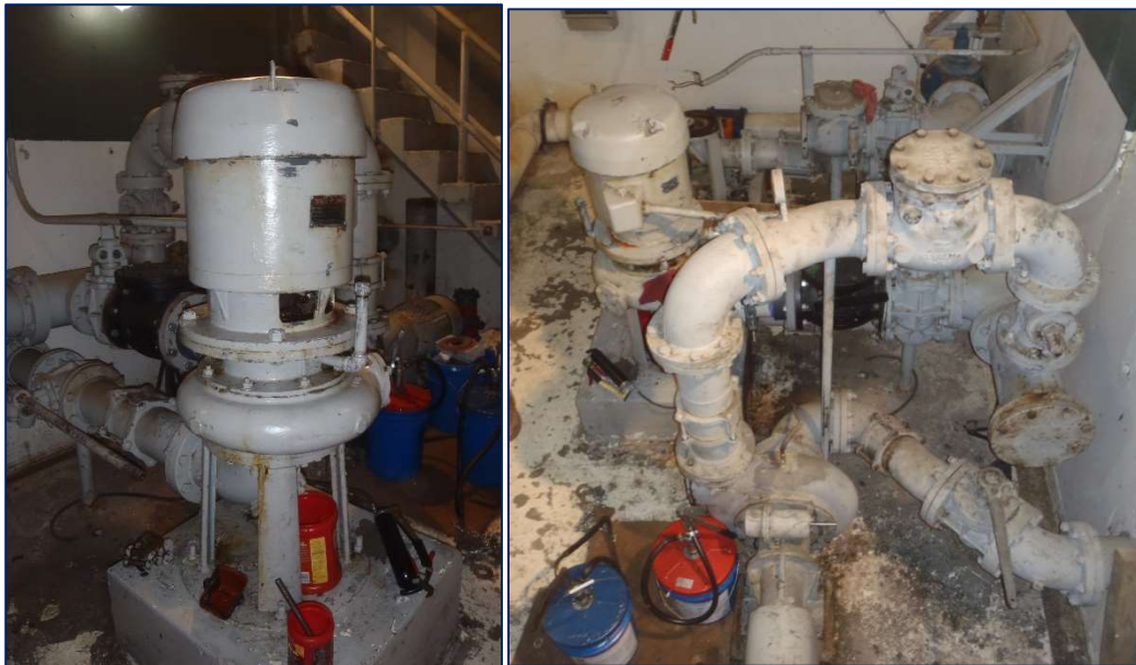
Figure 8. Influent pump station.
