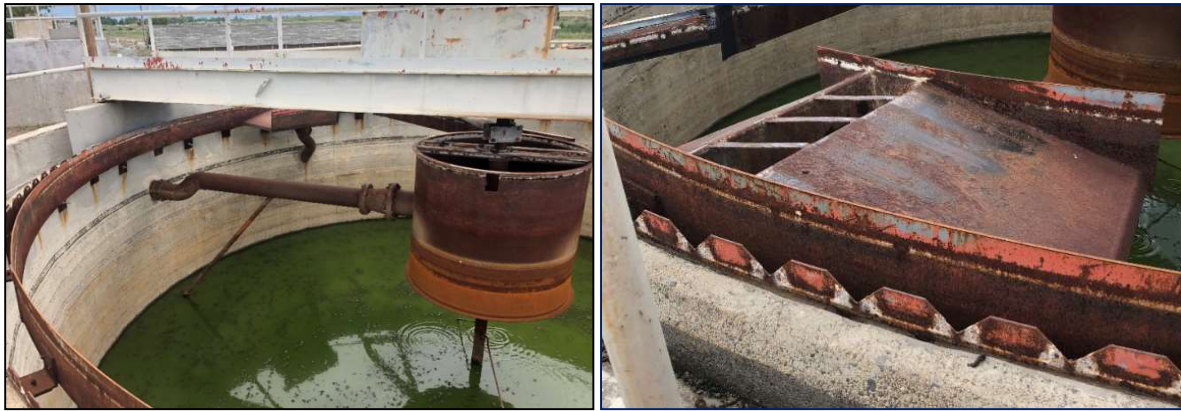
Figure 13. Secondary Clarifier #1 (currently offline).
