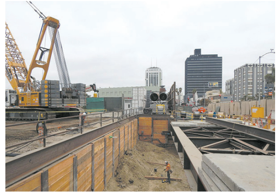
Coordination of underground utilities is critical to safely and efficiently operate Metro service.
