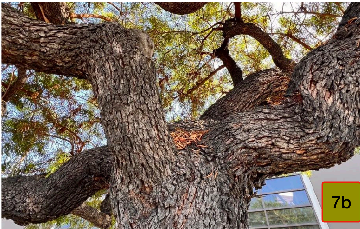
PHOTO - Shows City of Los Angeles street tree #7, recommended for removal and replacement. 7a, b) Represent poor structure and attachment for a tree of this species and size, that is prone to breakage. 8888 Venice Blvd, Los Angeles
