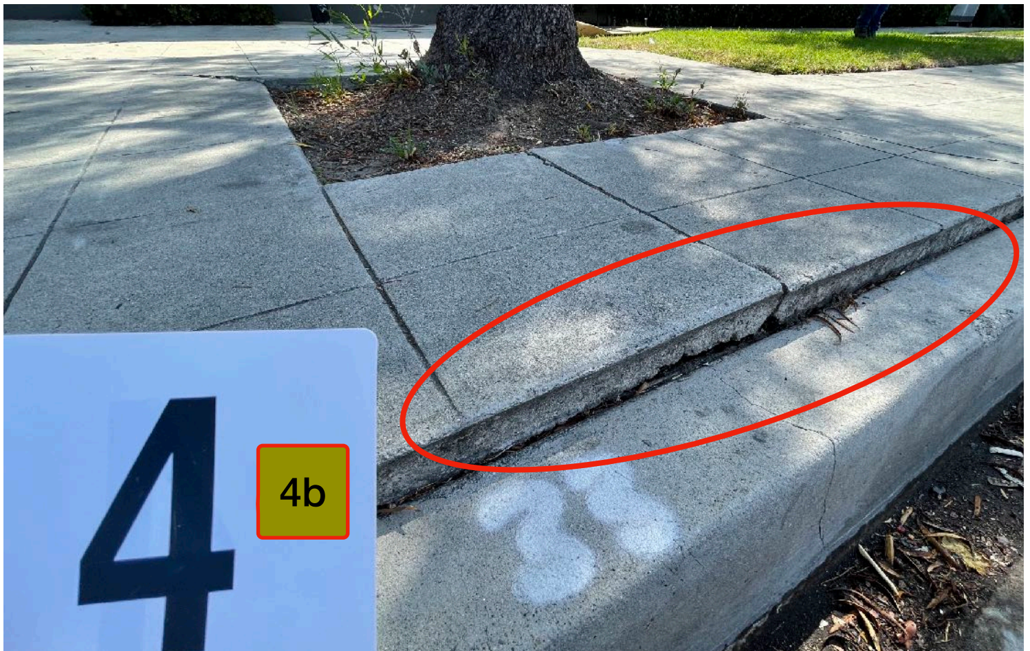
PHOTO - Shows City of Los Angeles street tree #4, recommend for removal.
